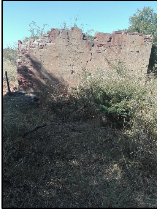
Figure 8: Dilapidated structure in Pella before split of Alternative Corridor 1 and Alternative Corridor 2 line.
