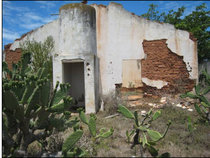
Aloedene – (S33 45 32; E 25 39.685) mostly demolished -2009 (Photo: P Martin)
