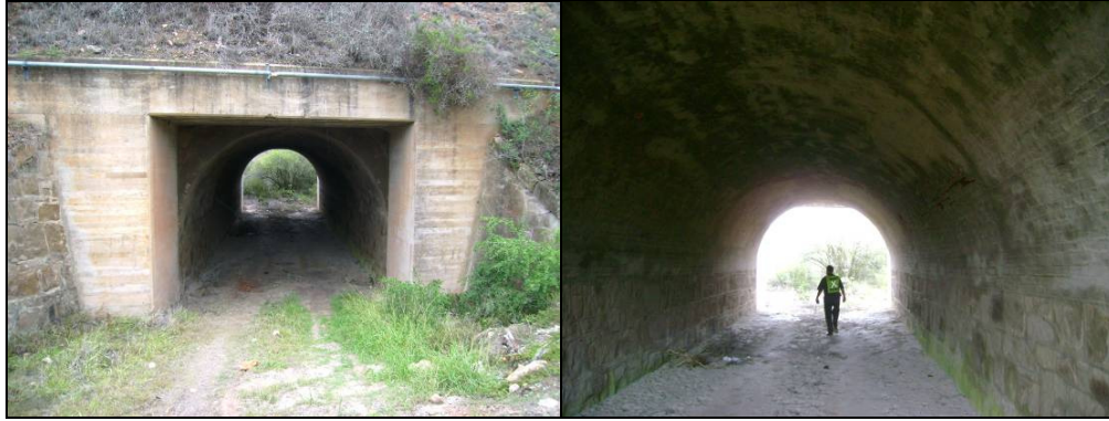
Stone viaduct—probably constructed when rail link to Uitenhage was built – c 1875 must be saved (see recommendations Section 12) S33 44.163; E25 40 043 (Photo JS Bennie)
