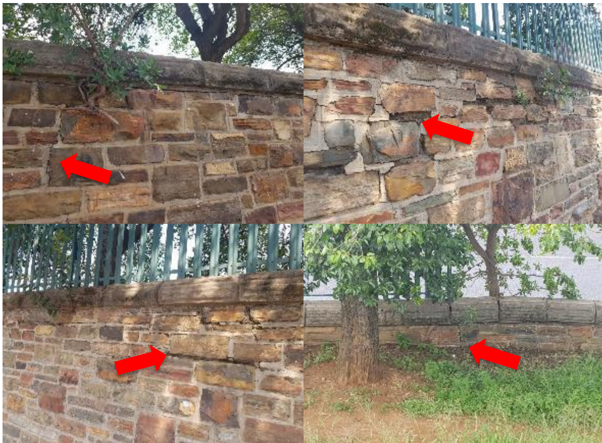
Figure 23: Cracks and breaks found along the Original Stone wall (Cracks indicated by red arrows – along Pretorius Street in the north)
