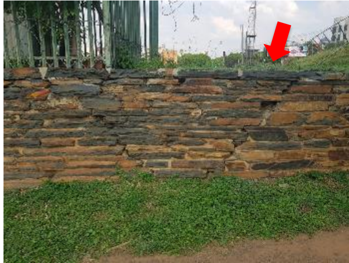
Figure 27: Cracked section (red arrow) in the smaller sandstone wall that needs to be repaired and conserved.
