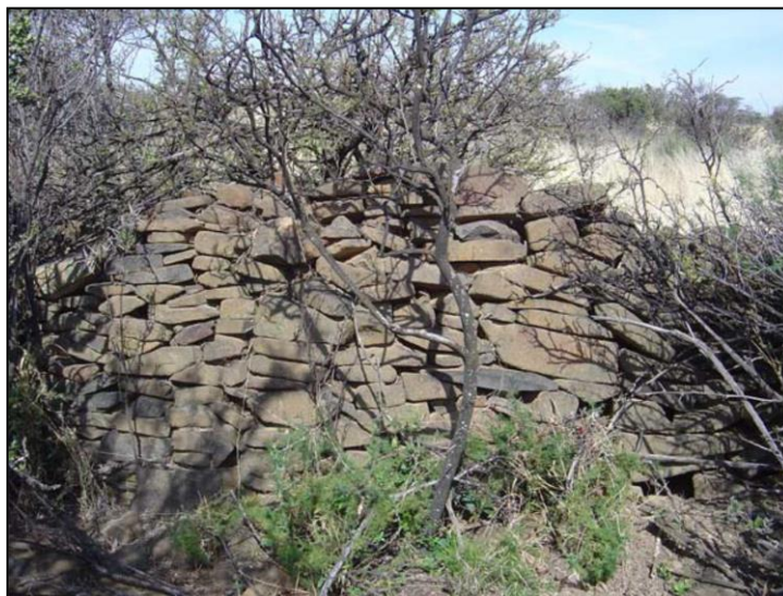
Figure 7-3: View of preserved Iron Age stone walling on the farm Middenspruit south of Kroonstad.
