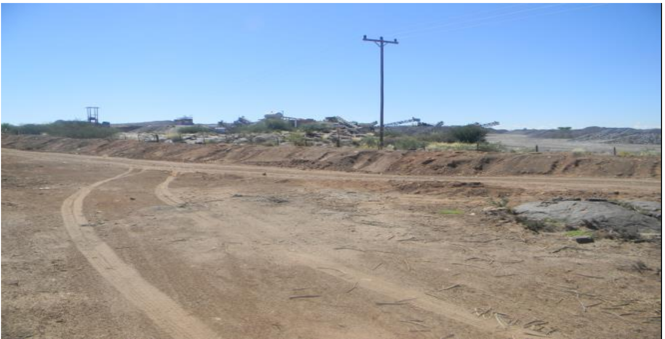
Plate 6: Photo 6: View of western section of the proposed development site (Photograph © by Author 2017).
