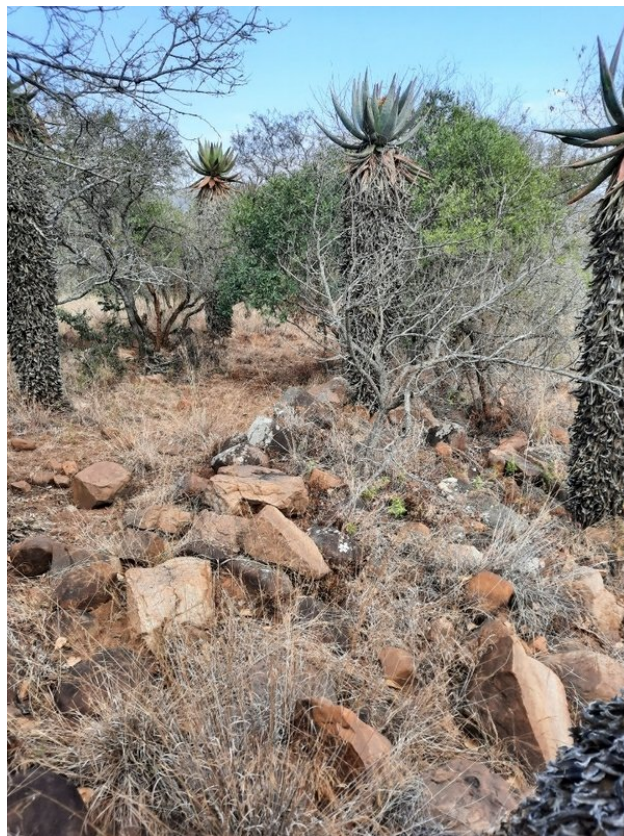
General site conditions - Degraded section of packed stone walling.
