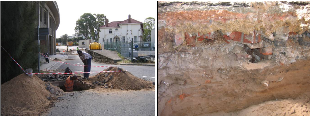
(l) Contractors test holes along the cable route in the Council Roads Depot off Ebenezer Road (r) Large amounts of rubble fill were noted in the upper parts of the holes overlying in situ sandy deposits.
