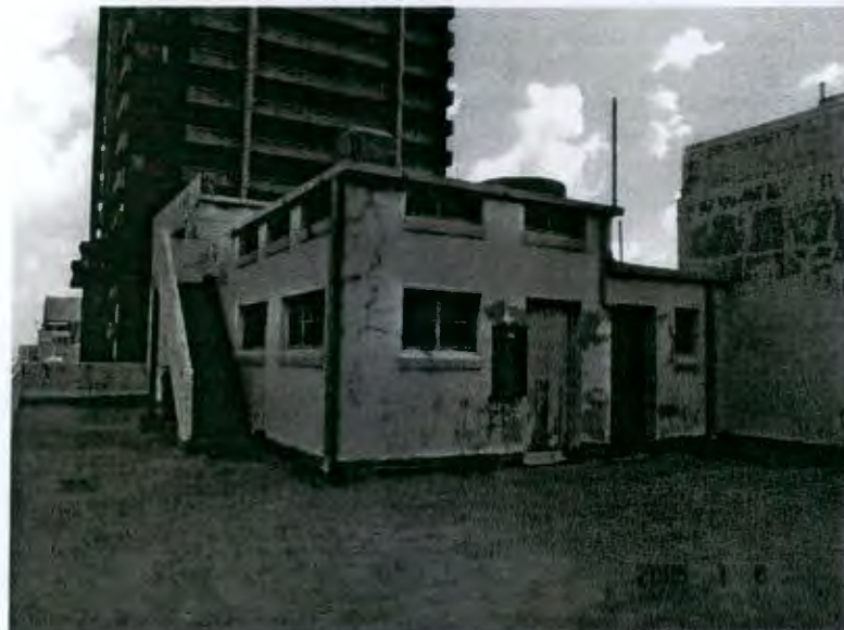
Close-up view of the service accommodation and lift motor room on top of Clegg House
