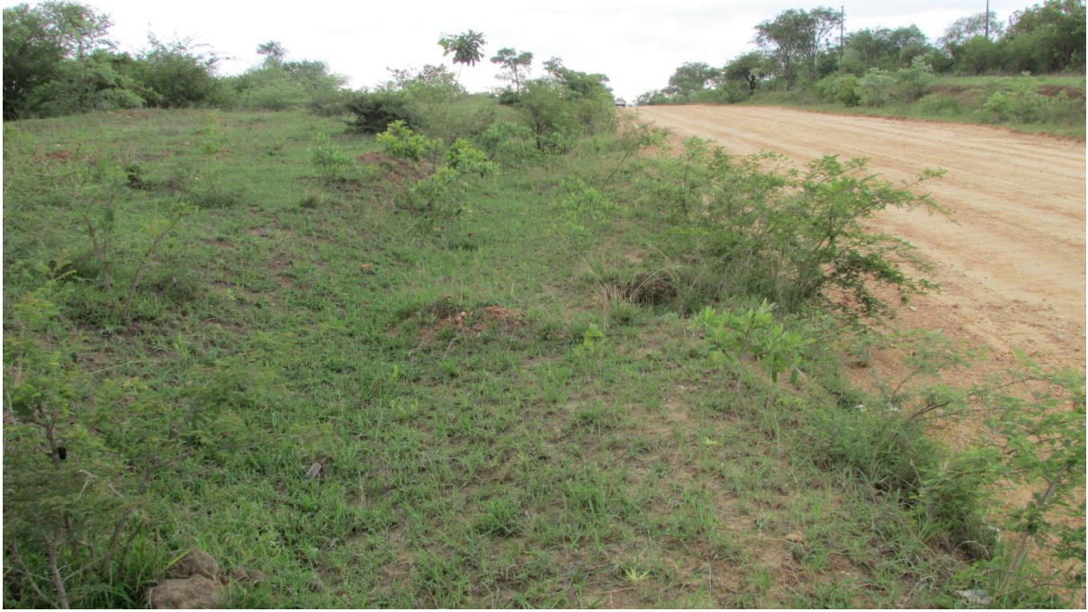
Figure 5: View of some of the section of the road upgrade, note the bumpy patch on the side of the road. This has vehemently caused the disturbance.
