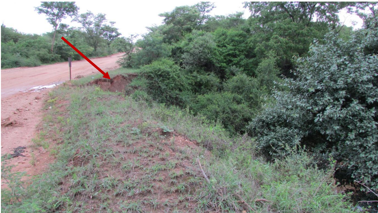
Figure 14: An overview of the southern section of the bridge to be refurbished, note the collapse as indicated by the arrow.
