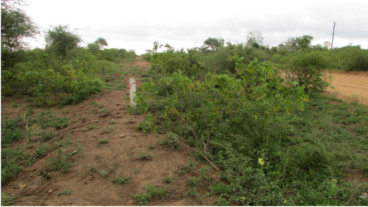
Figure 11: An overview of the side of the road, note the disturbance caused by the water pipeline installation.
