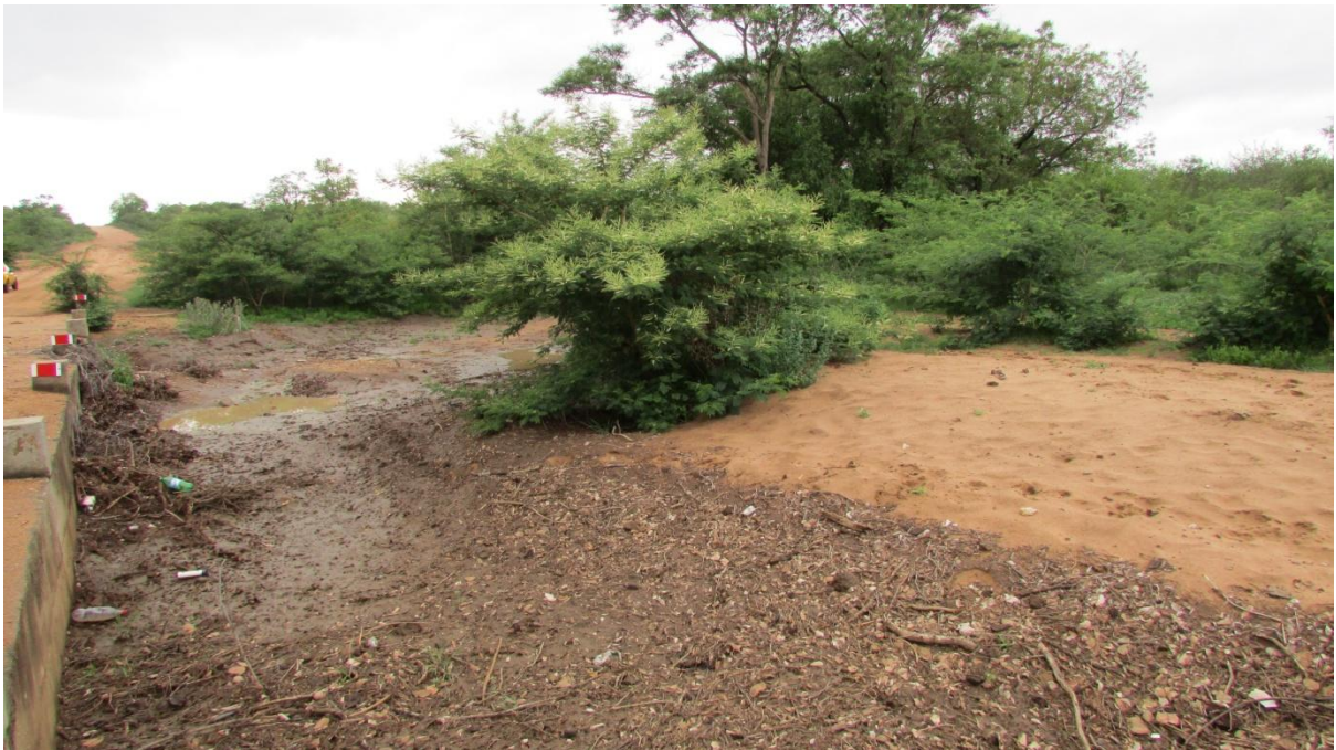
Figure 18: View of the southern section of the culvert proposed to be refurbished.
