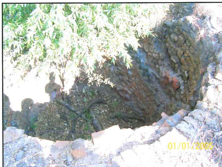
Fig 10: Lime-burning kiln showing refractory brick and vegetation which is causing damage to the brick lining
