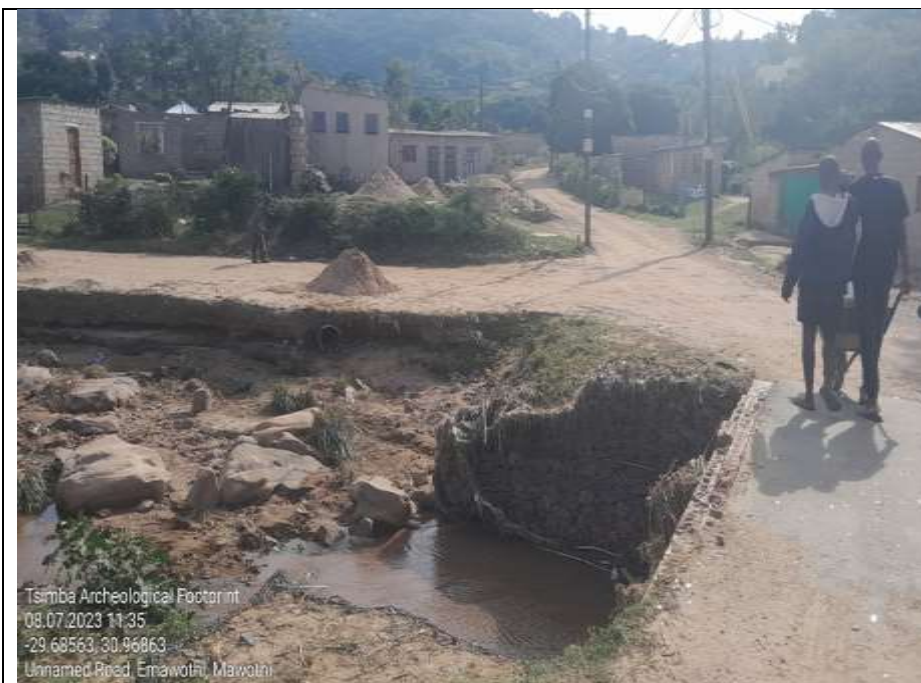
Figure 4: View of the starting point the sewer collector, visible is the Ohlanga River and the bridge structure
