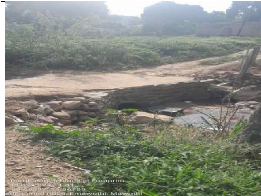
Figure 8: View of a river stream and bridge along the proposed sewer pipeline route
