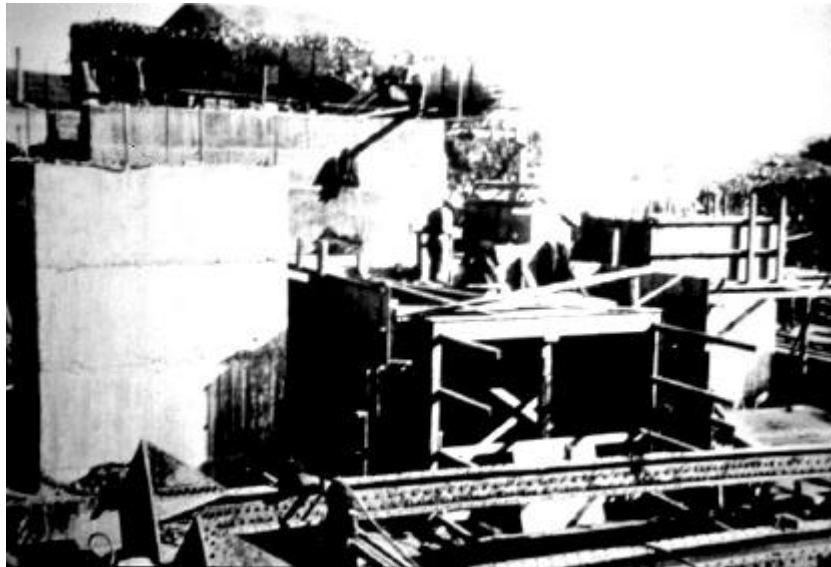
Figure 7: Building the grain elevator – “View of track shed, hoppers and tunnels, with working house. Columns laying horizontal ready to lift into place. Columns are 47' long and weigh approx 9 tons each.” 22 (ref: DW0201)
