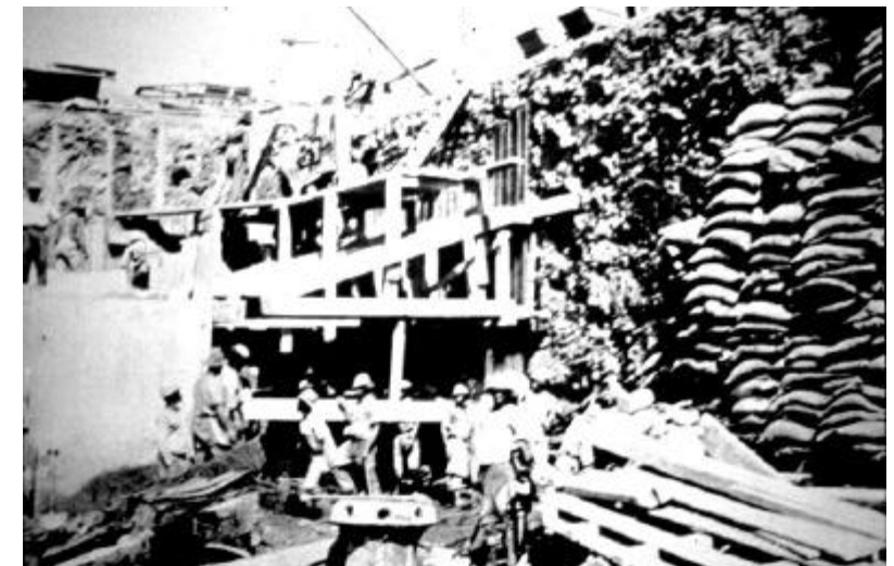
Figure 6: Building the grain elevator - "you will notice the ship's capstan in this photo, this being the position where the wreck was." 21 (ref: DW0193)
