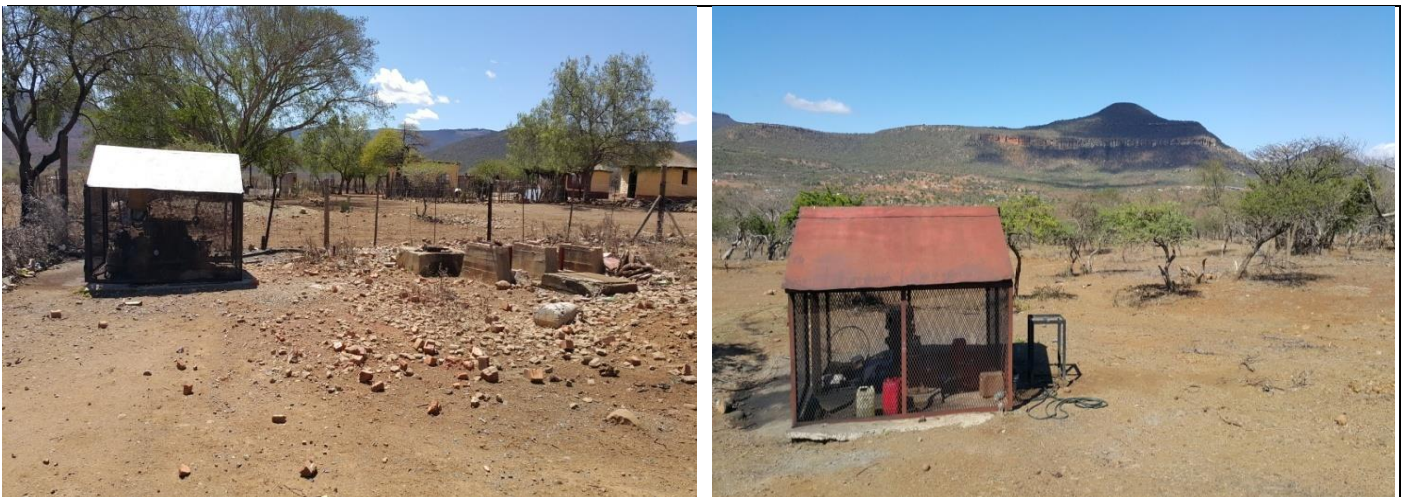
Figure 10- Diesel engines that assist with pumping of water from reservoirs and boreholes to communities
