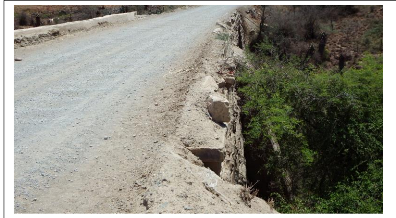
Figure 7: The bridge carriageway showing missing side safety walls. (Photo: The Author)
