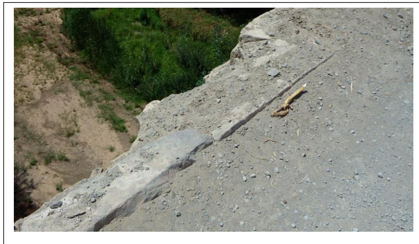
Figure 6: Missing side safety wall. (Photo: The Author)
