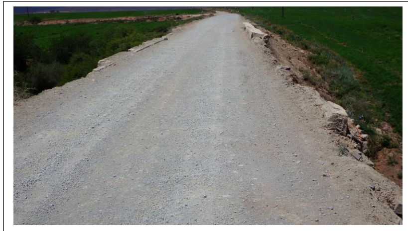
Figure 5: The bridge carriageway. Note the missing safety walls. (Photo: The Author)
