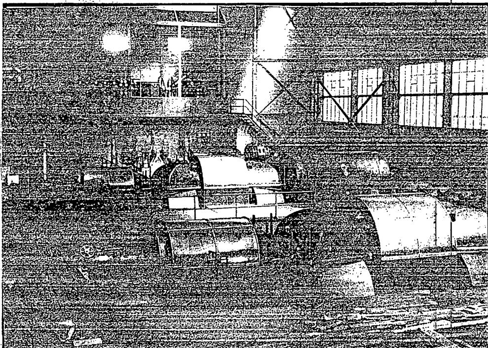
B) View in Turbine House, looking southwards, showing No's.1 and 2 Parsons' 20'000KW Sets and Parsons' 1'000KW auxiliary turbo alternator (near south wall), sine anno (VFTP, no number).
