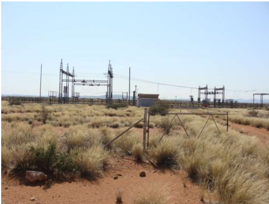
Figure 5 The Fibre Substation.
