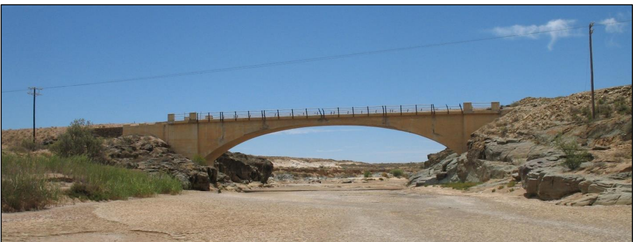
Figure 20: View of the old single-span road bridge over the Sout River [4 February 2008].
