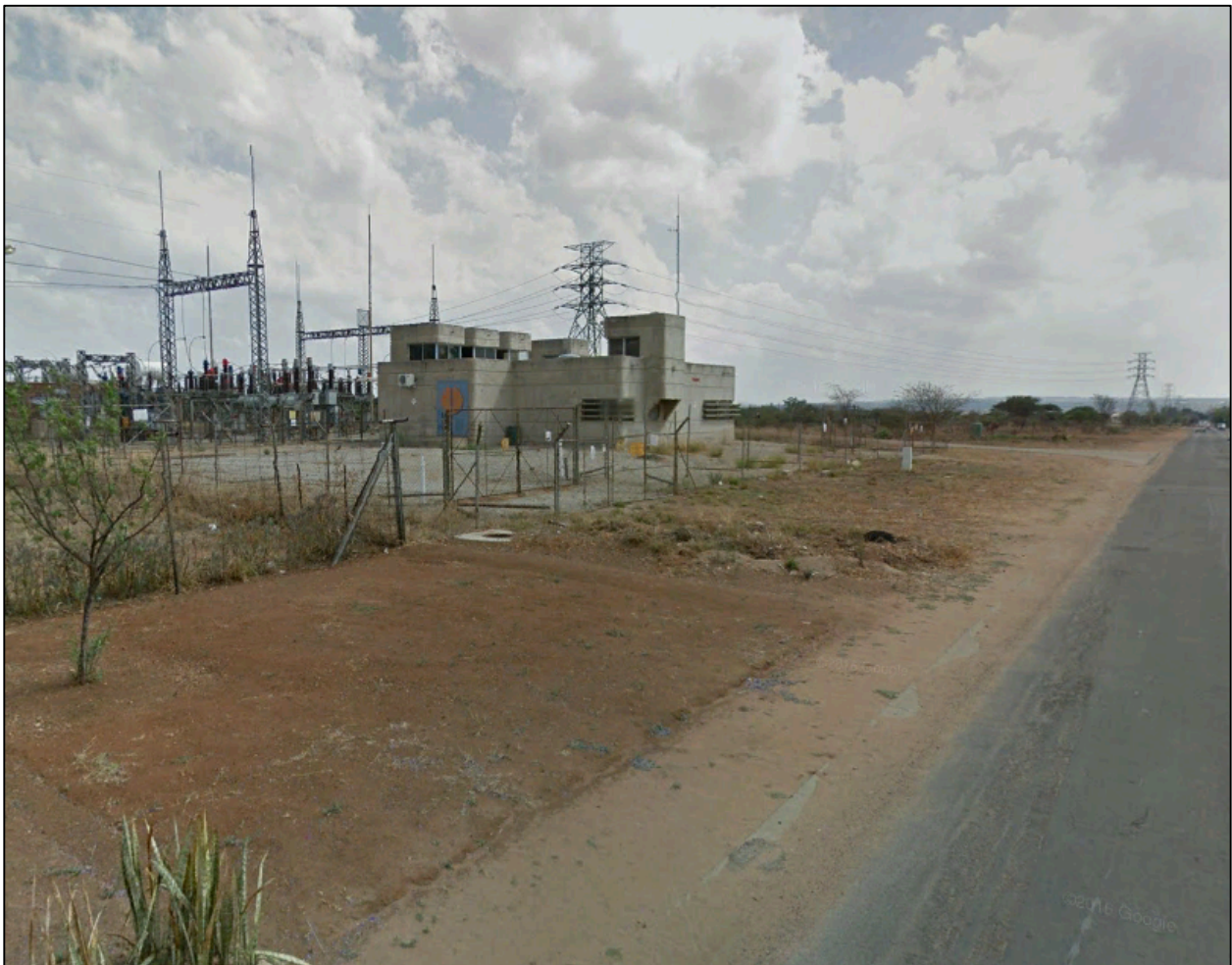
Figure 8. Substation located on Railway Street, Polokwane
