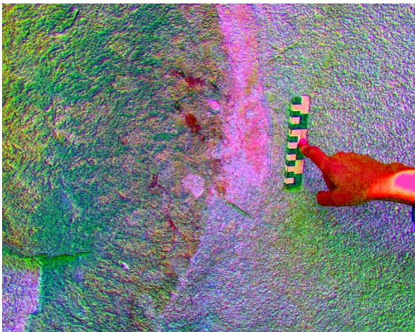
Fig. 15: Seep marks obscure these images.
