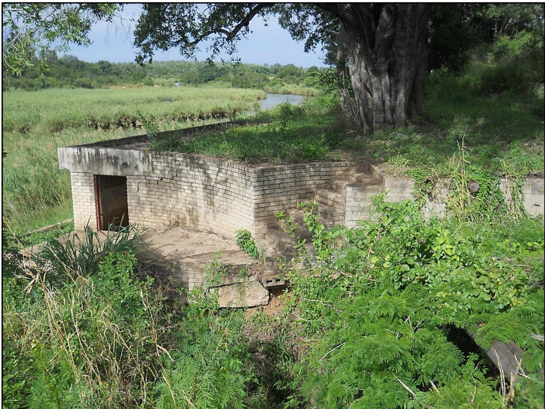
Figure 2. View of the existing abandoned abstraction station with Sabie River in the background.
