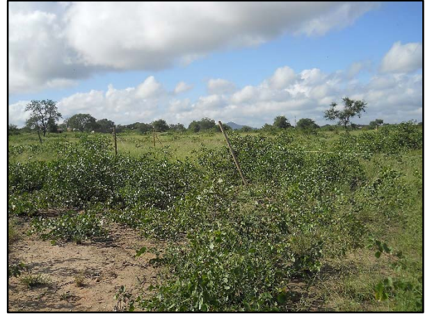
Figure 2. Bush clearance and plot preparation in the central-western section – photo taken in south-easterly direction
