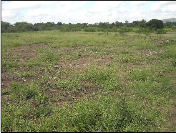
Figure 1. Bush clearance and plot preparation in the southern section – photo taken in southerly direction
