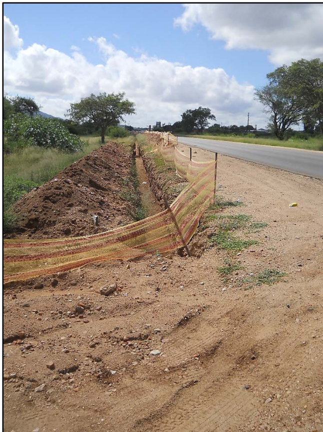
Figure 2. View of the cable trench along the northern shoulder of the road in an easterly direction.
