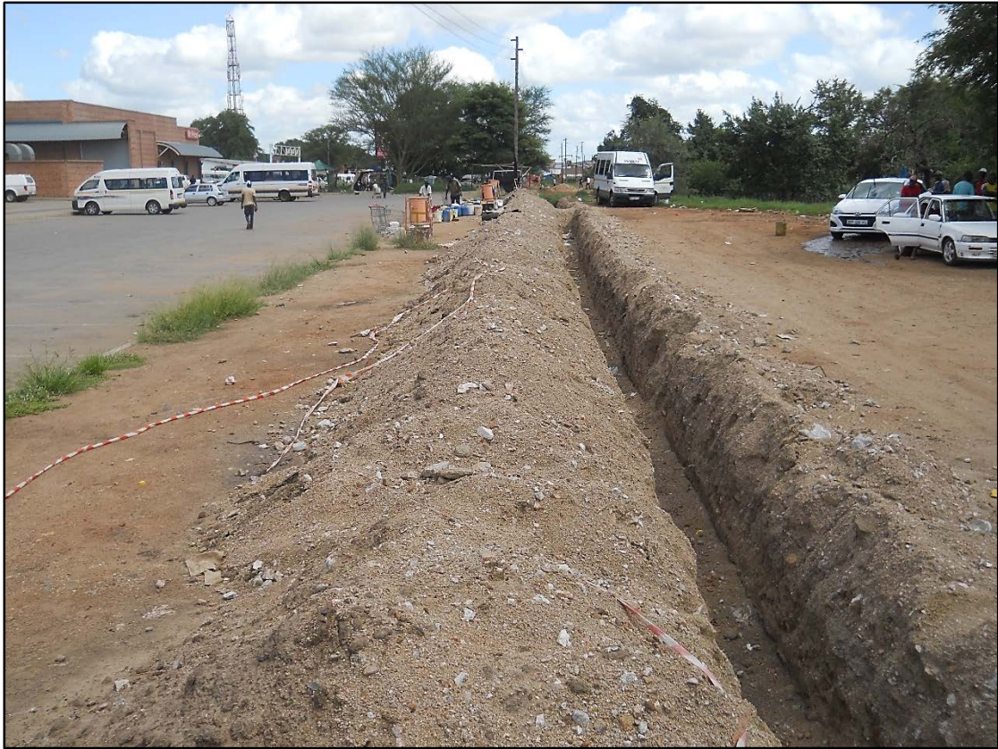
Figure 7. View of the cable trench passing a Taxi stand – westerly direction.
