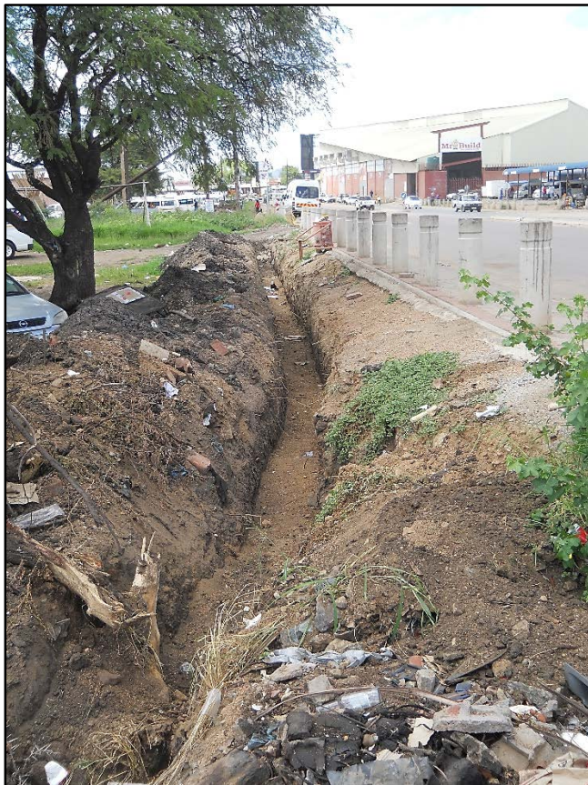
Figure 6. View of the cable trench along First Street in the CBD – easterly direction.
