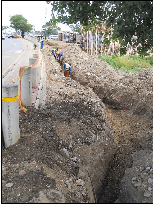
Figure 5. View of the cable trenching by hand along First Street – westerly direction.
