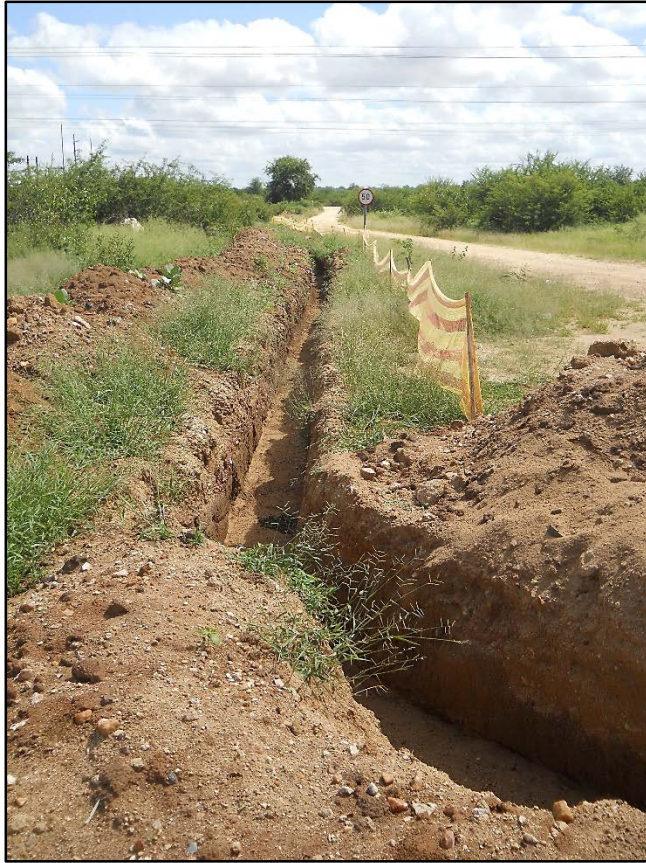
Figure 1. View of the cable trench from the road to the Eskom substation. Northerly direction
