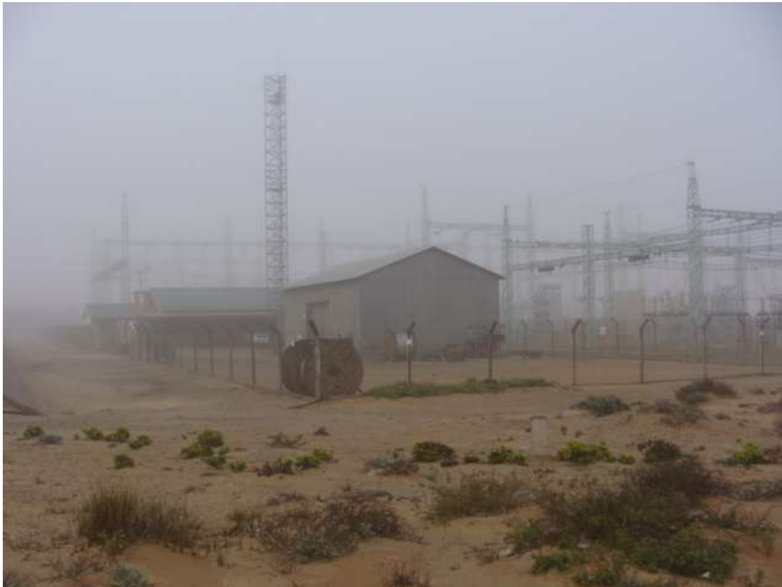
Figure 19: The existing substation in the surveyed area.
