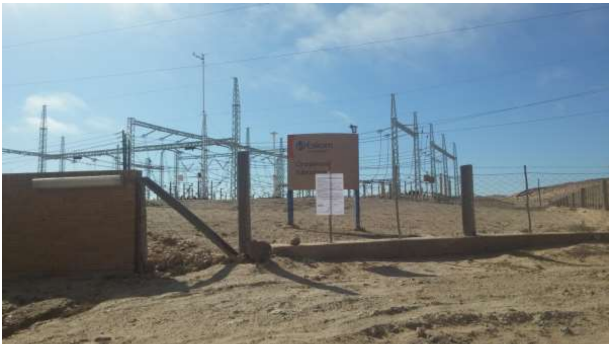
Figure 8: Site notice at the Oranjemond substation.
