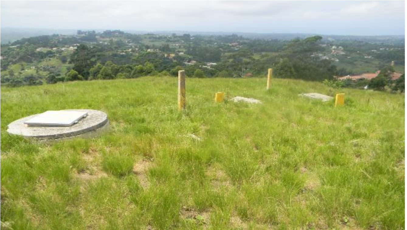
Plate 3: Photo 3: View of existing pipeline and water reticulation infrastructure which are earmarked for upgrading (Photograph © by Author 2017)
