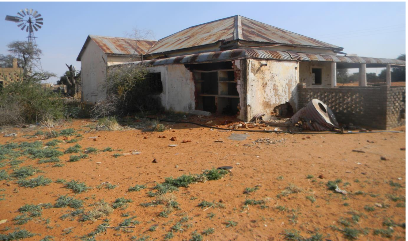
Plate 28: showing derelict facades of a historic farmhouse.
