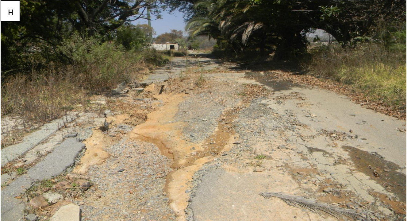
Plate 9: Photo H, Showing dilapidated road within the proposed development site.
