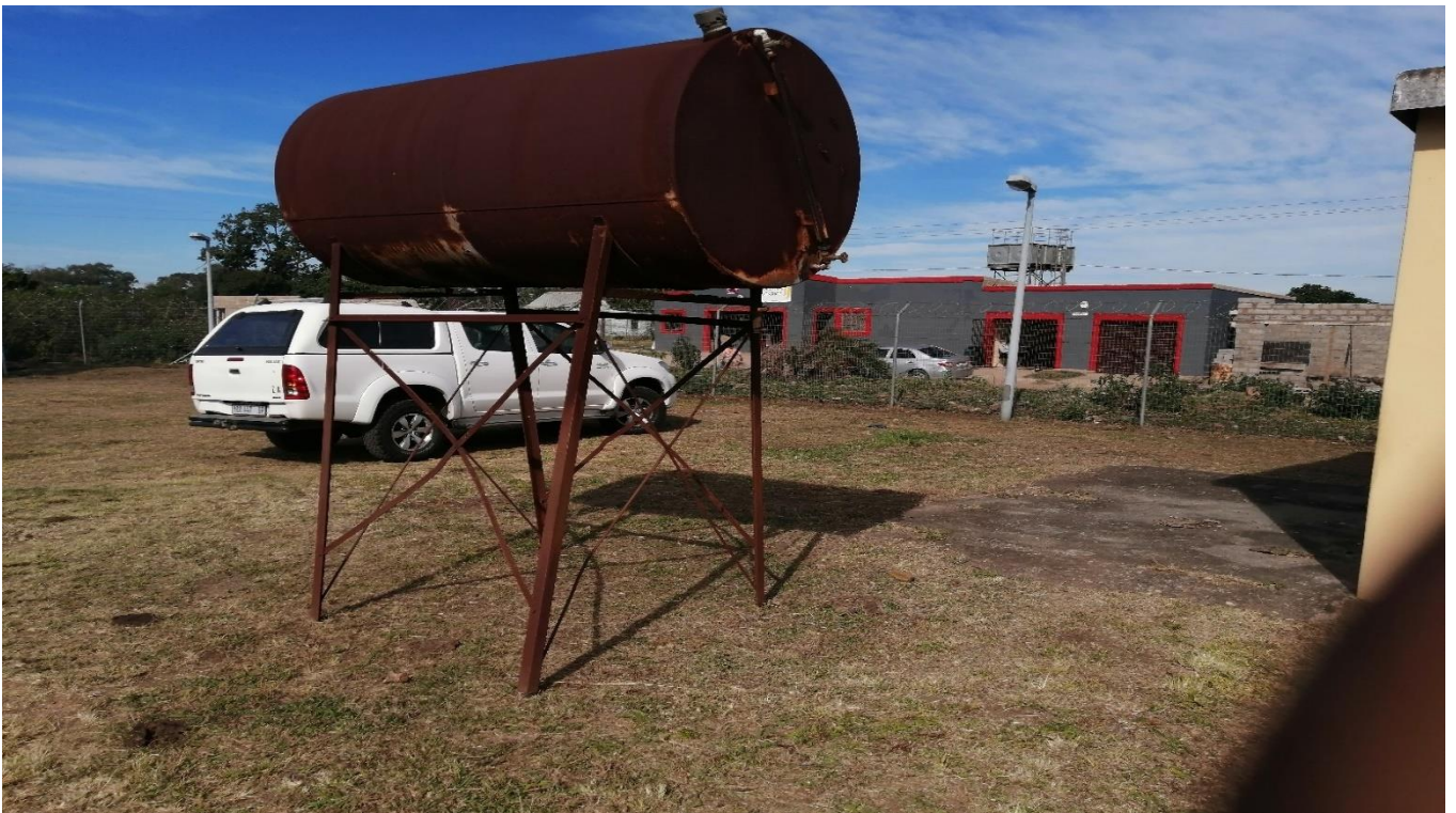
Plate 4: Showing an elevated fuel tank in its delapidated state within the proposed development site
