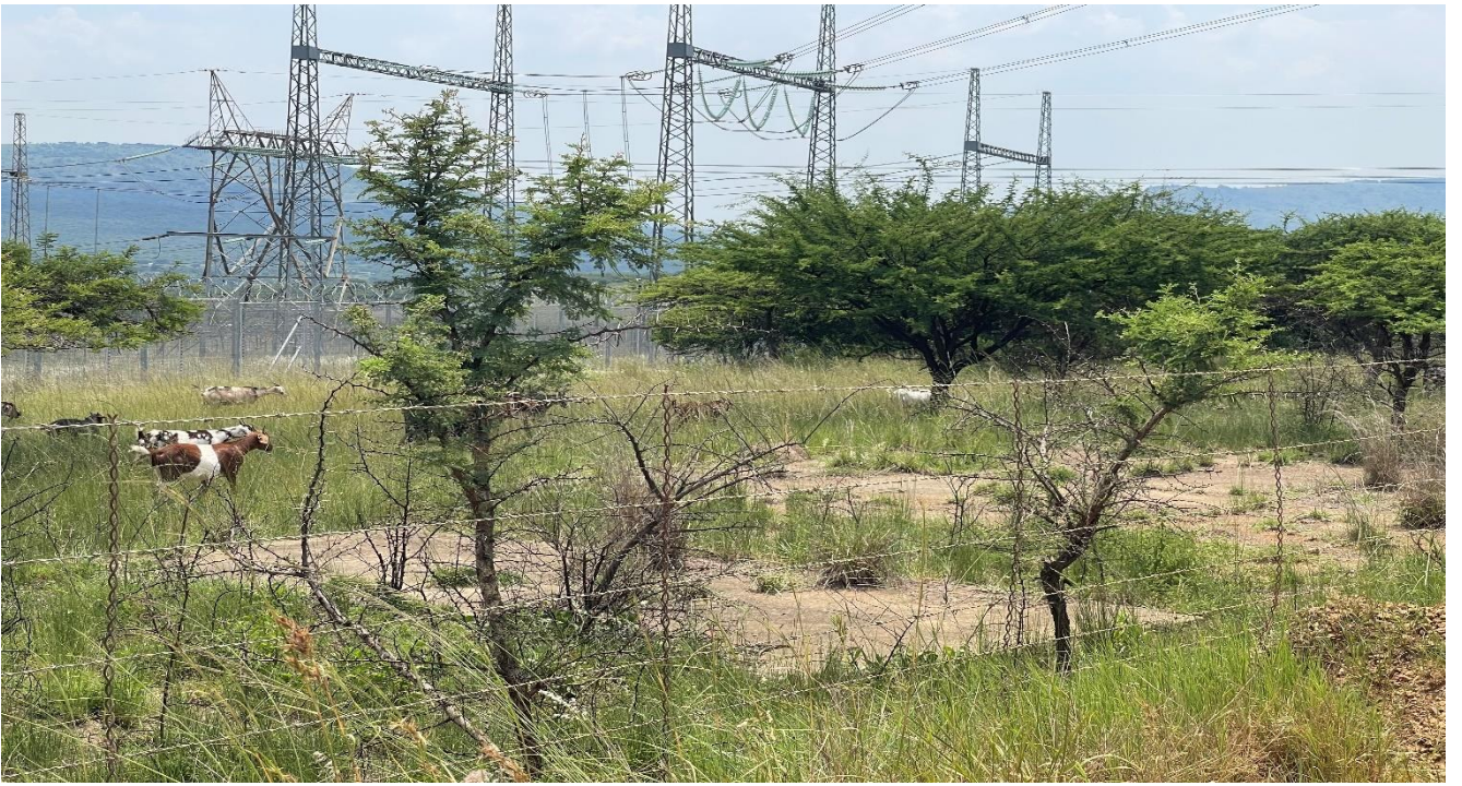
Plate 2: showing the Umfolozi Substation
