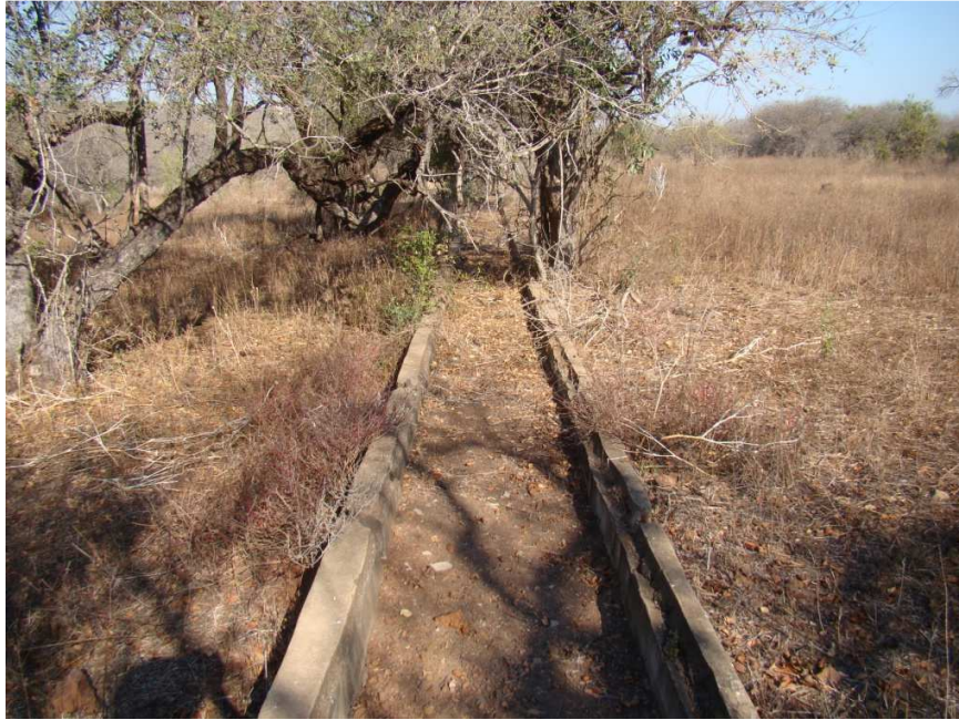
Fig. 19: A neglected concrete water canal runs towards the pump house.
