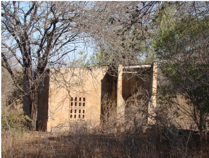
Fig. 18: A neglected pump house is located in Block B near a drainage line.
