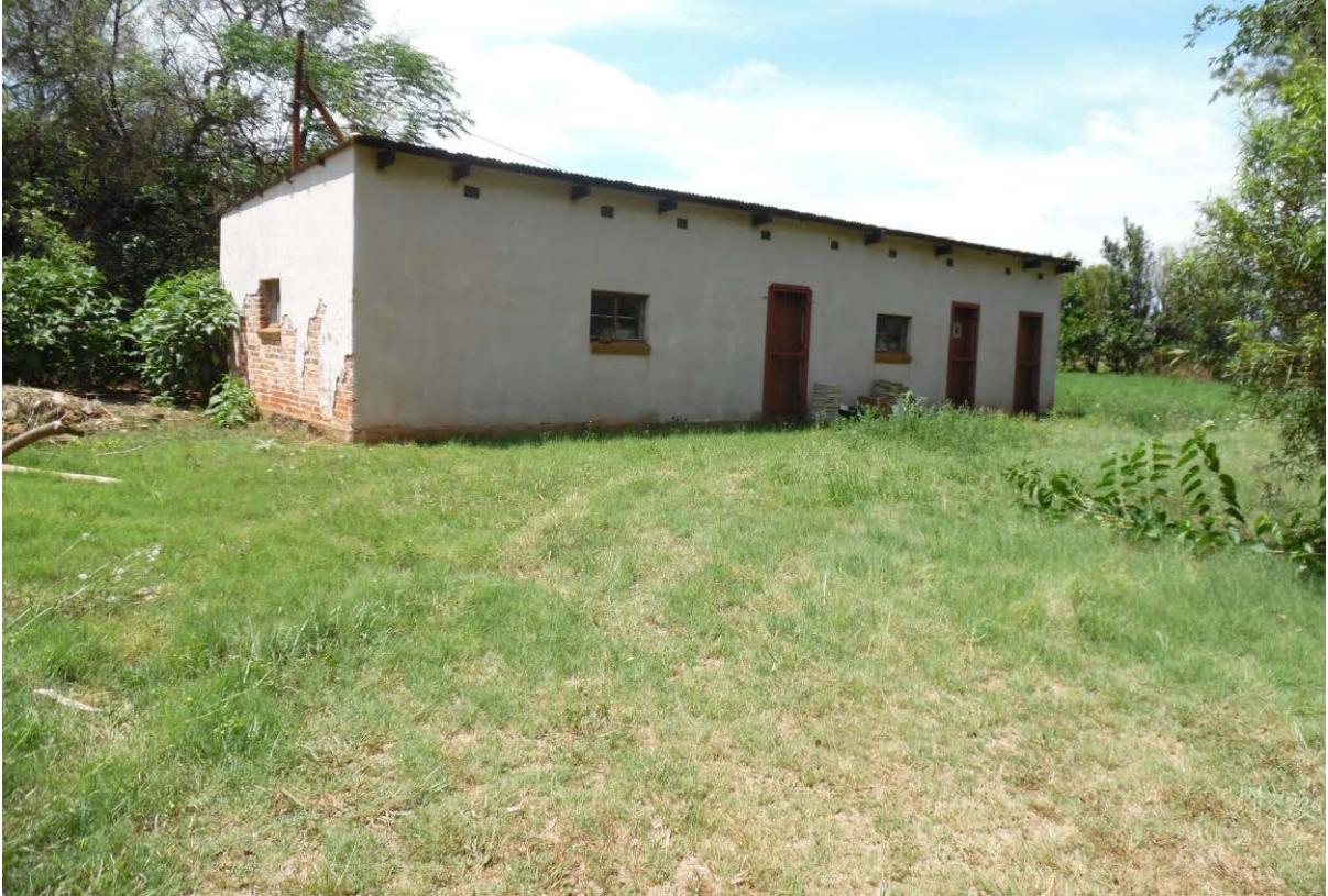
Figure 14: Structure older than 60 years. During the Public Participation Process (PPP) this structure was identified as a structure constructed by Italian Prisoners of War
