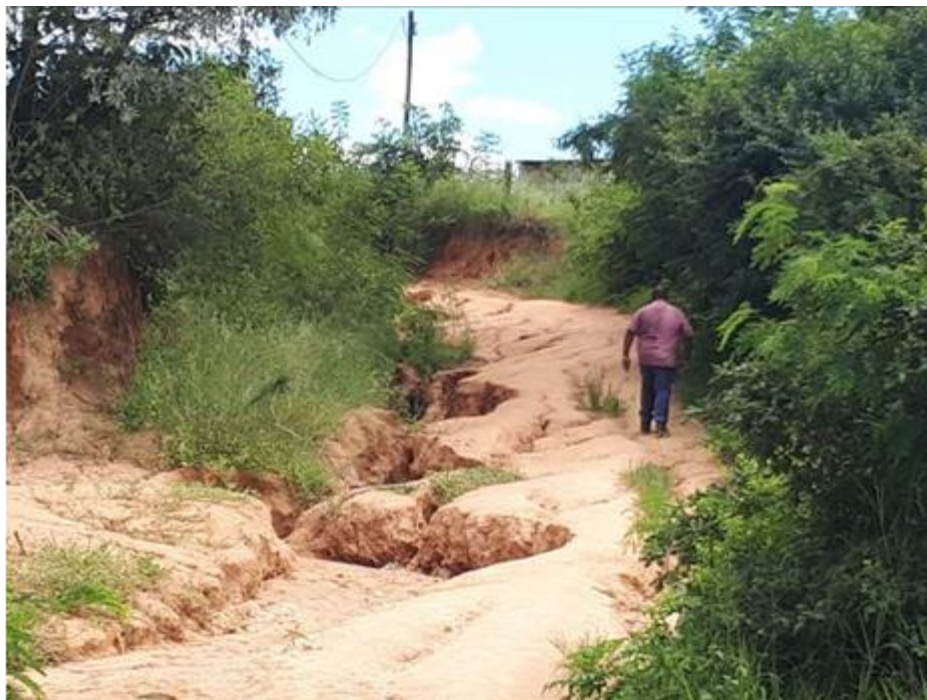
Fig. 31: The general condition of the road further east, towards point D (courtesy AFRIKA Enviro & Biology).
