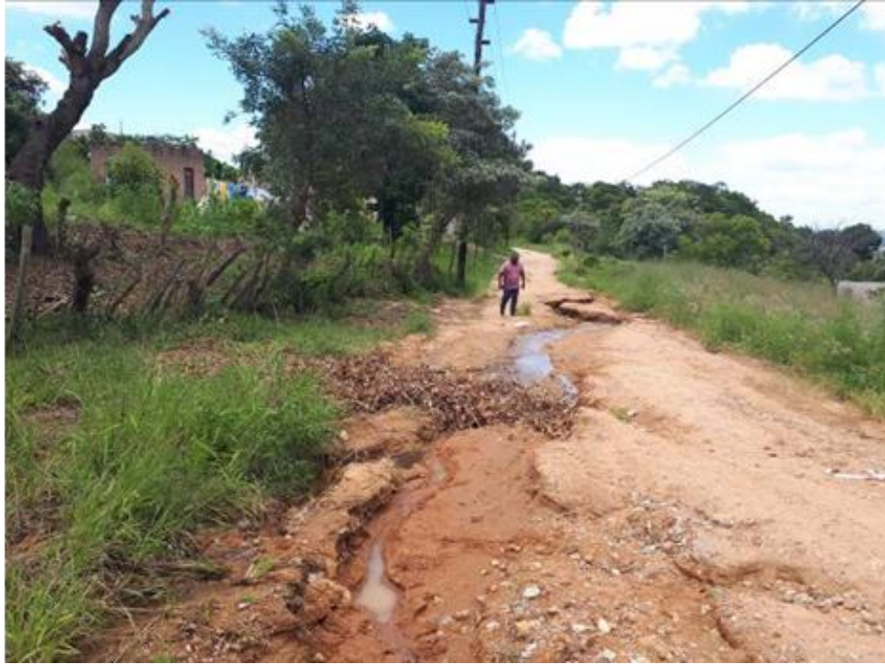
Fig. 32: The proposed upgrading of the roads will greatly improve living conditions in the residential area where most of the informal roads are severely eroded (courtesy AFRIKA Enviro & Biology).
