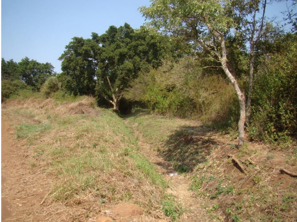
Fig. 29: A drainage line which was dug out to form a canal, starts in section D.
