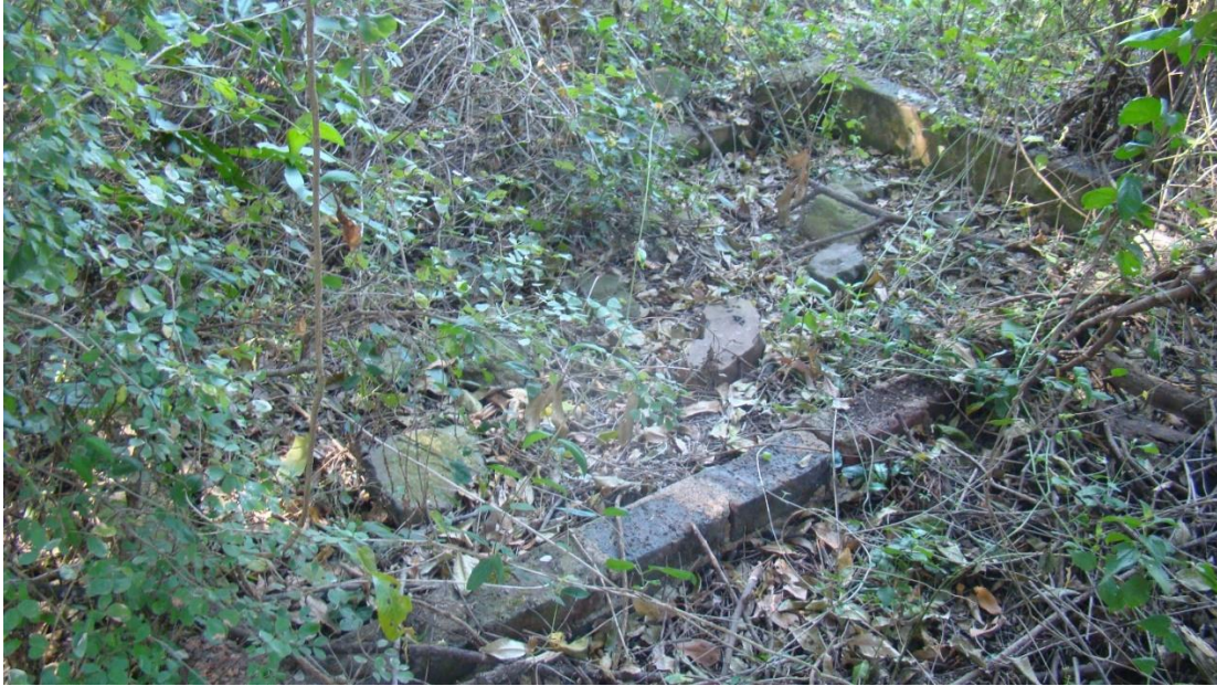
Fig. 21: An overgrown square foundation of approximately 2500mm x 1500mm was observed near the river. The bricks are modern and recent and it is believed to be the foundation of an earlier pump house.
