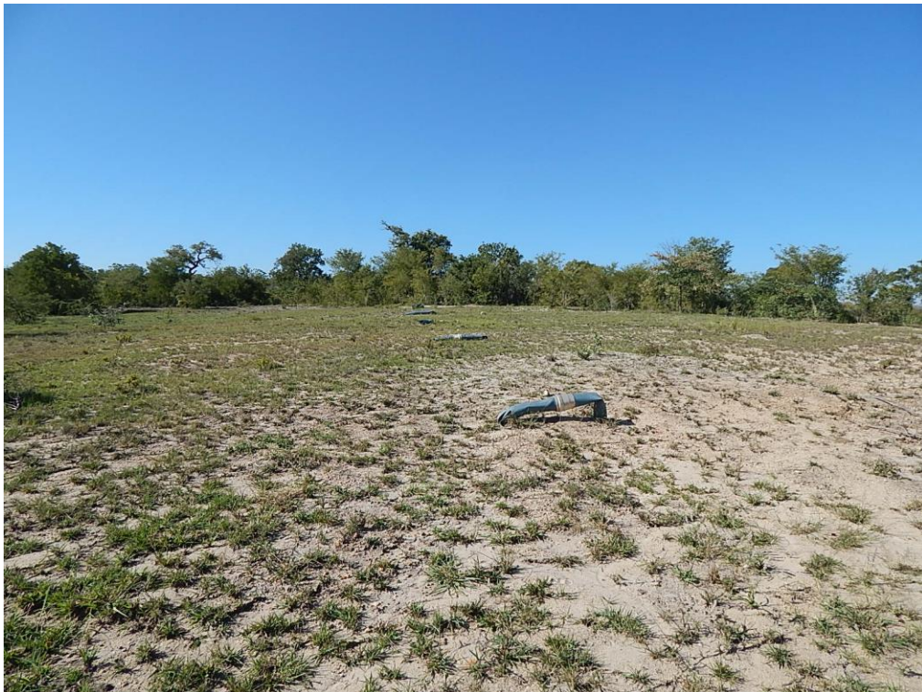
Fig. 10: Old pipeline infrastructure which formed part of the water reticulation for the historically cultivated lands (south-eastern section).
