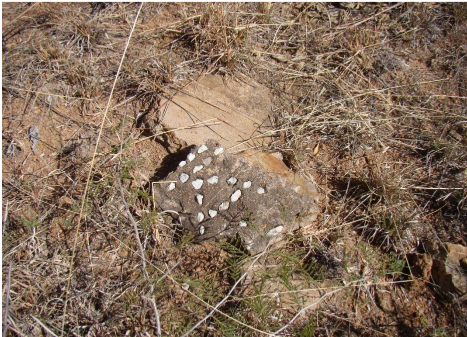
Fig. 6: Concrete foundation with a section which contains a pattern of small white pebbles.
