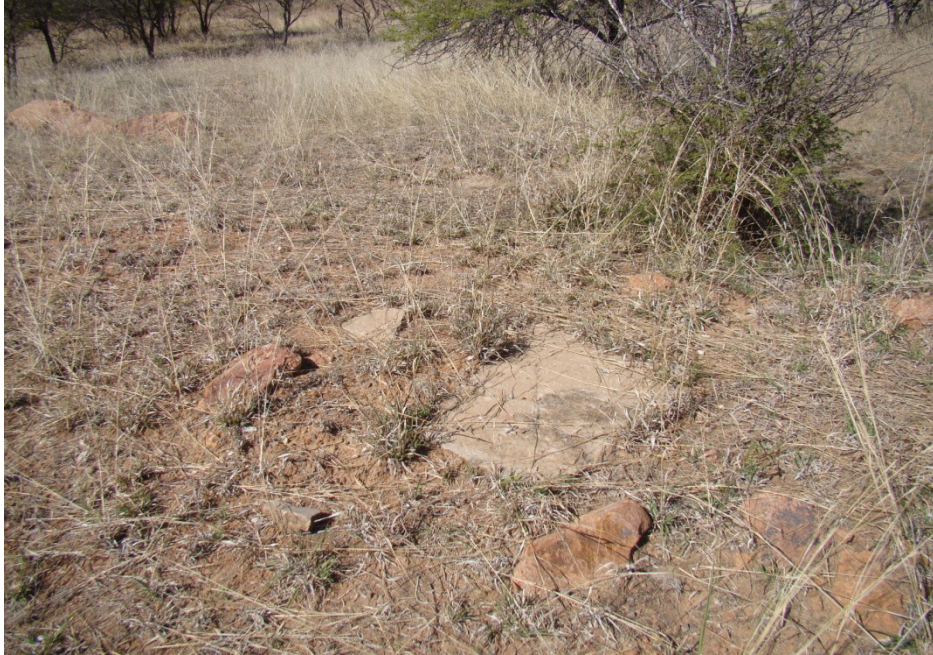
Fig. 5: Remains of a foundation. Concrete, stones and bricks of a recent structure.
