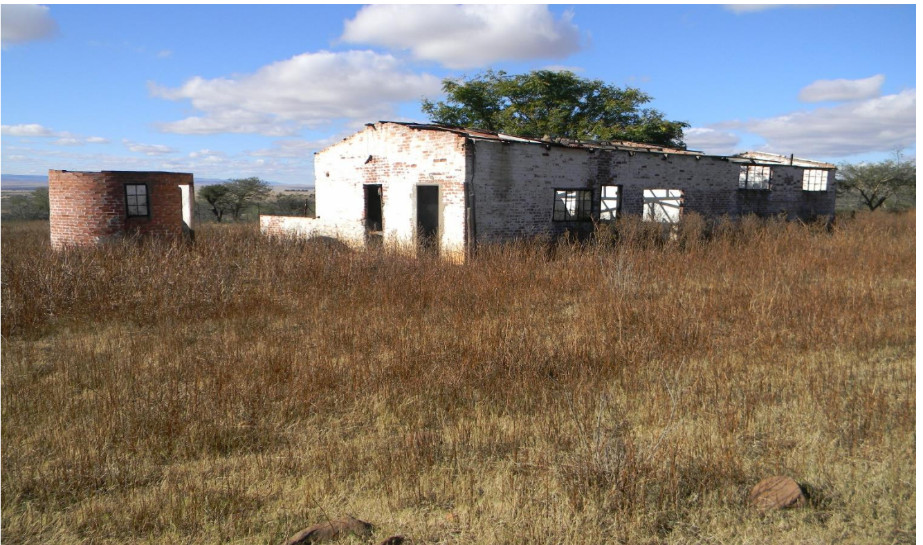
Plate 60: showing a vandalised farm house which is probably more than 60 years old.
