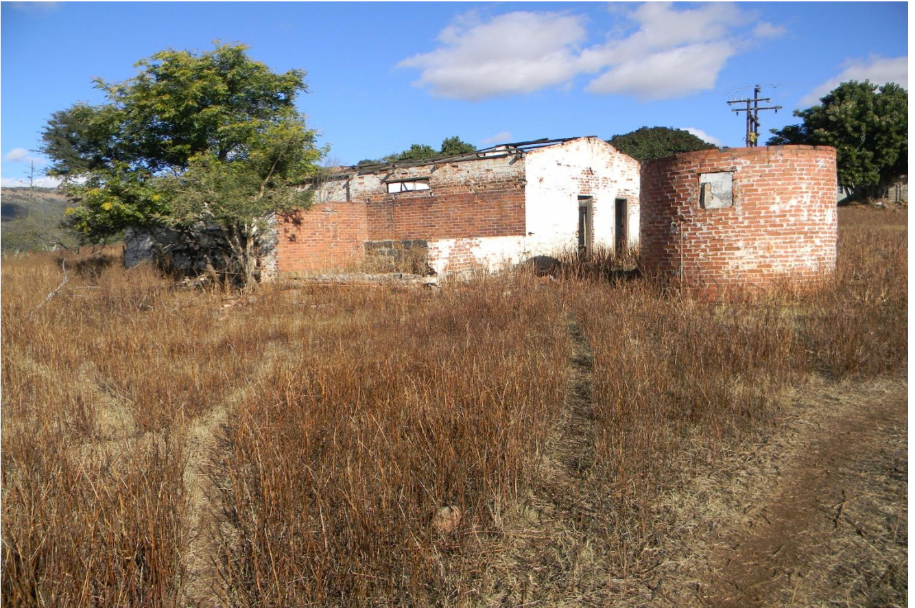
Plate 61: showing a vandalised farm house which is probably more than 60 years old.
