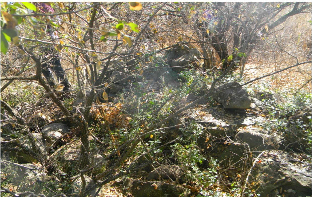
Plate 48: showing stone walls disturbed by vegetation overgrowth.
