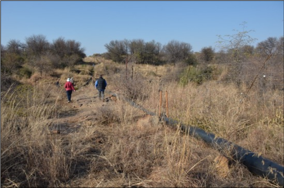
Figure 11. Pipeline at the Bierspruit Crossing
