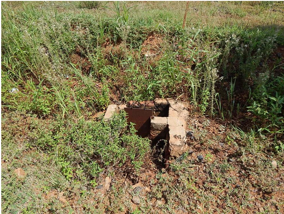
Fig. 14: Several sluices are visible within the earth canal to regulate water, on the study area.
