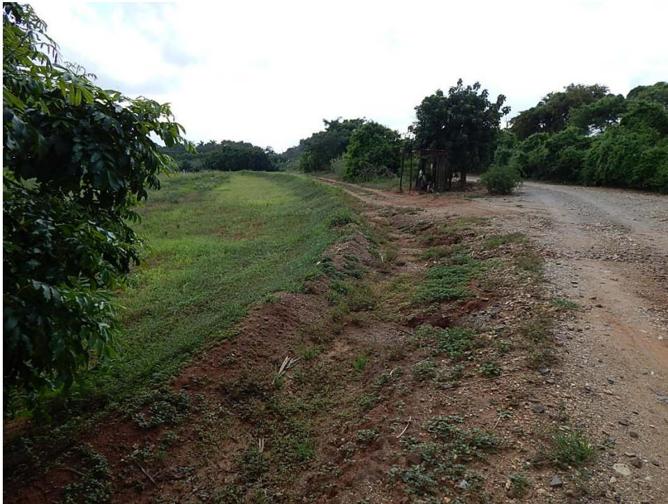
Fig. 22: The earth canal in the eastern section is visible next to the gravel road, facing east.
