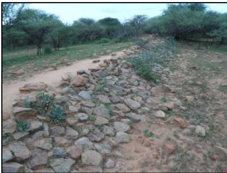
Figure 70 - Dam. Note the stone cladding to support the soil layer of the dam
