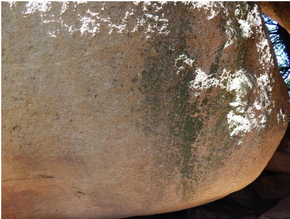
Fig. 48: Water seepage and lichen growth is seen towards the far right of the panel (1A).
