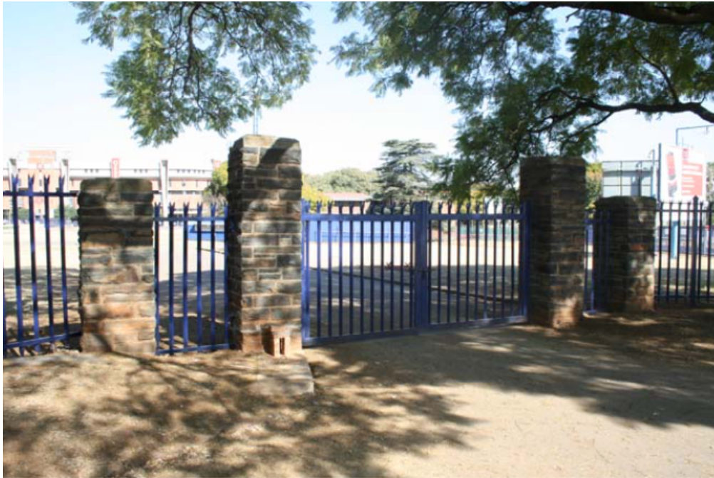
Figure 15 The Entrance gate on the corner of Park and Kirkness Streets. (F Coetzee, 2012)
