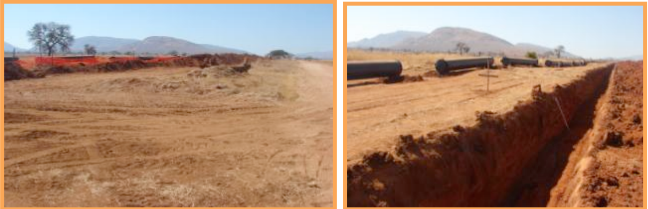
Plates 4 and 5: Pictorial view of the Platreef loop in and out powerline route (Left) and bulk water pipeline servitude currently under construction running parallel to the proposed Platreef loop in and out powerline route (Right).
