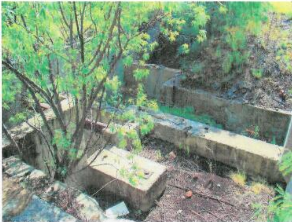
Figure 35: Detail of the concrete channels and sub-surface chambers at the "Crushers" area (4)
