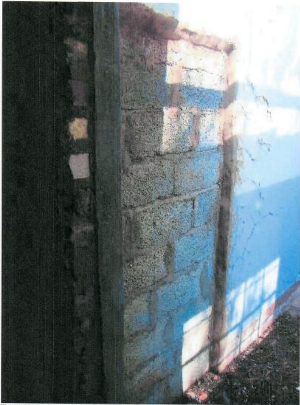
Figure 42: Blocked up entrance to tunnel that connects compound to the change room and the change room to the mine (situated on the western side of the Change Room)
