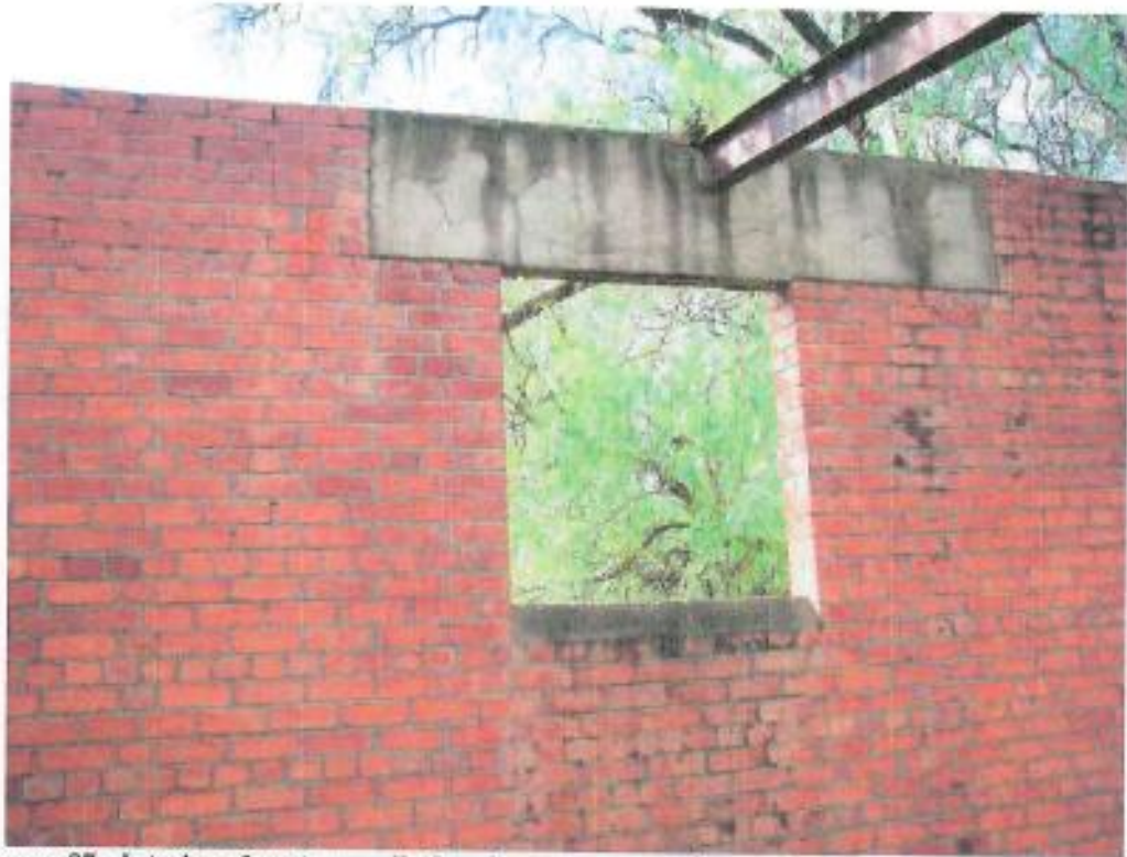
Figure 97: Interior of western wall of engine room – metal beam that connected the engine room with the shaft
