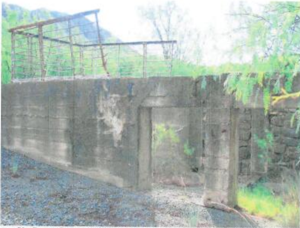
Figure 91: Cement Structure which probably served as foundation for the shaft gear (Modern Tailings Dump in background). Orientation south-west.
