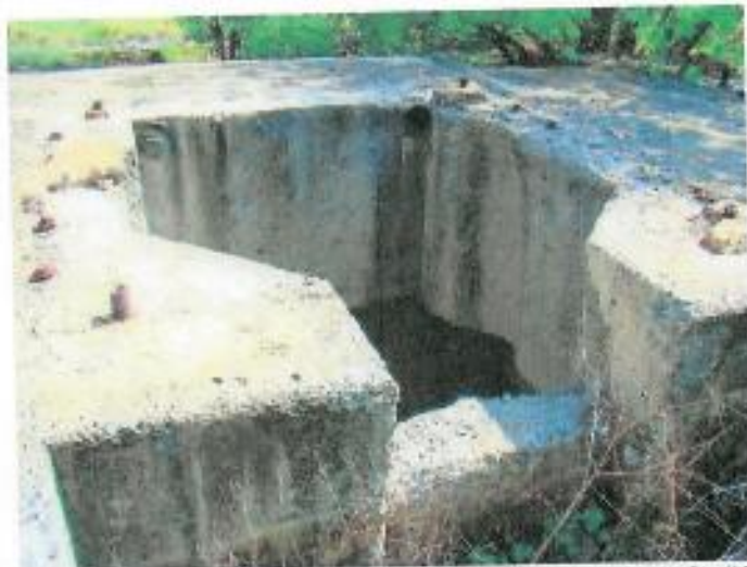
Figure 33: Detail of the sub-surface concrete channels and chambers at the "Crushers" area (2)
