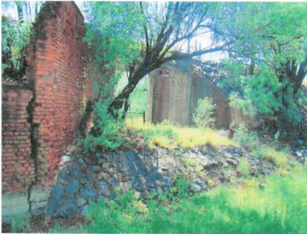
Figure 60: The brick reinforced section curves north-east towards an opening in the wall (cement-constructed bridge)
