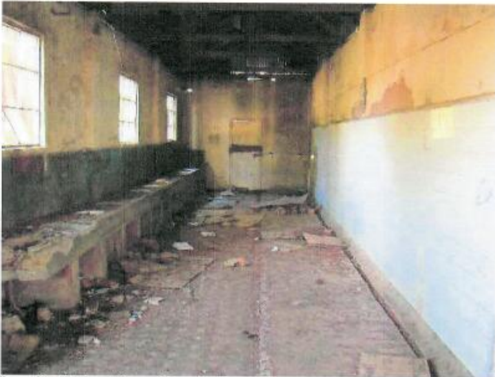
Figure 40: Interior of Change House that is connected to the southern side of the Shaft Offices (western section)
