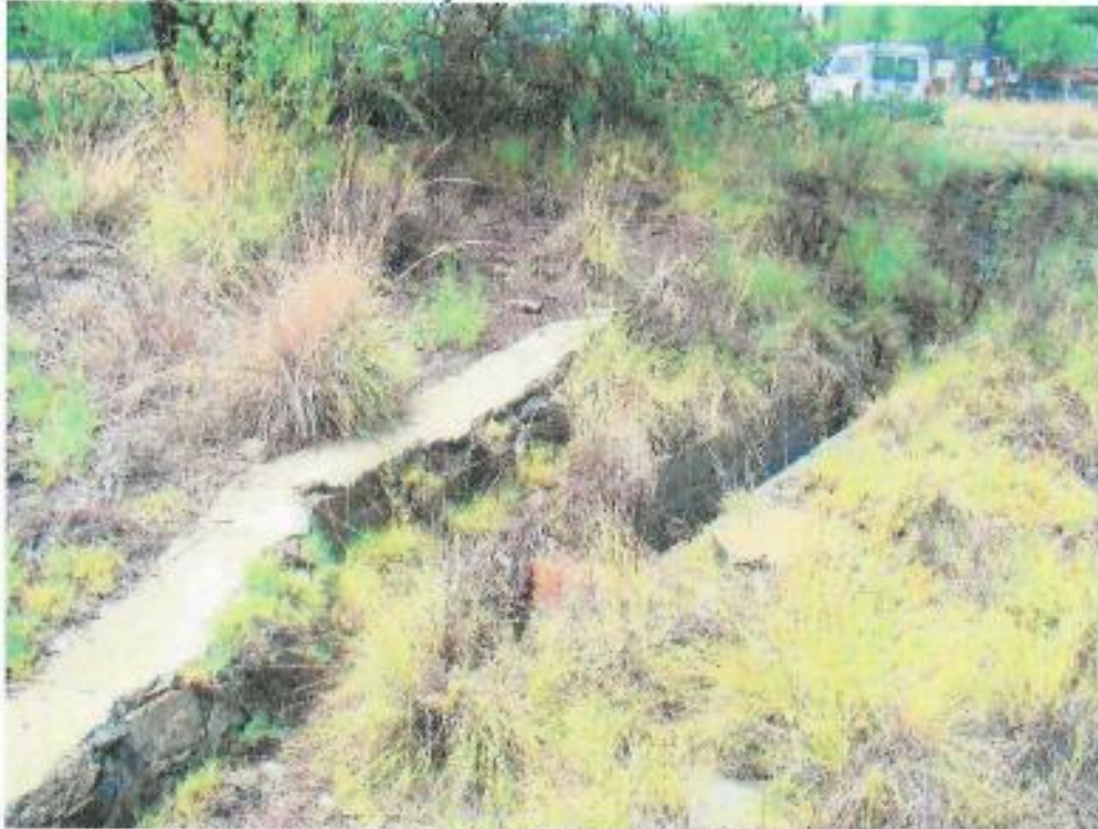
Figure 53: Remains of foundation of unknown structure with ditch on side (south-easterly orientation)
