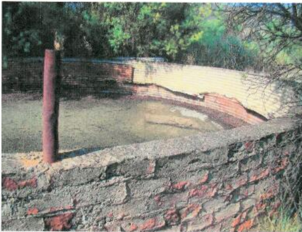
Figure 82: Detail of raised dam in picture 36 above - constructed of bricks & mortar and lined with sheets of corrugated iron
