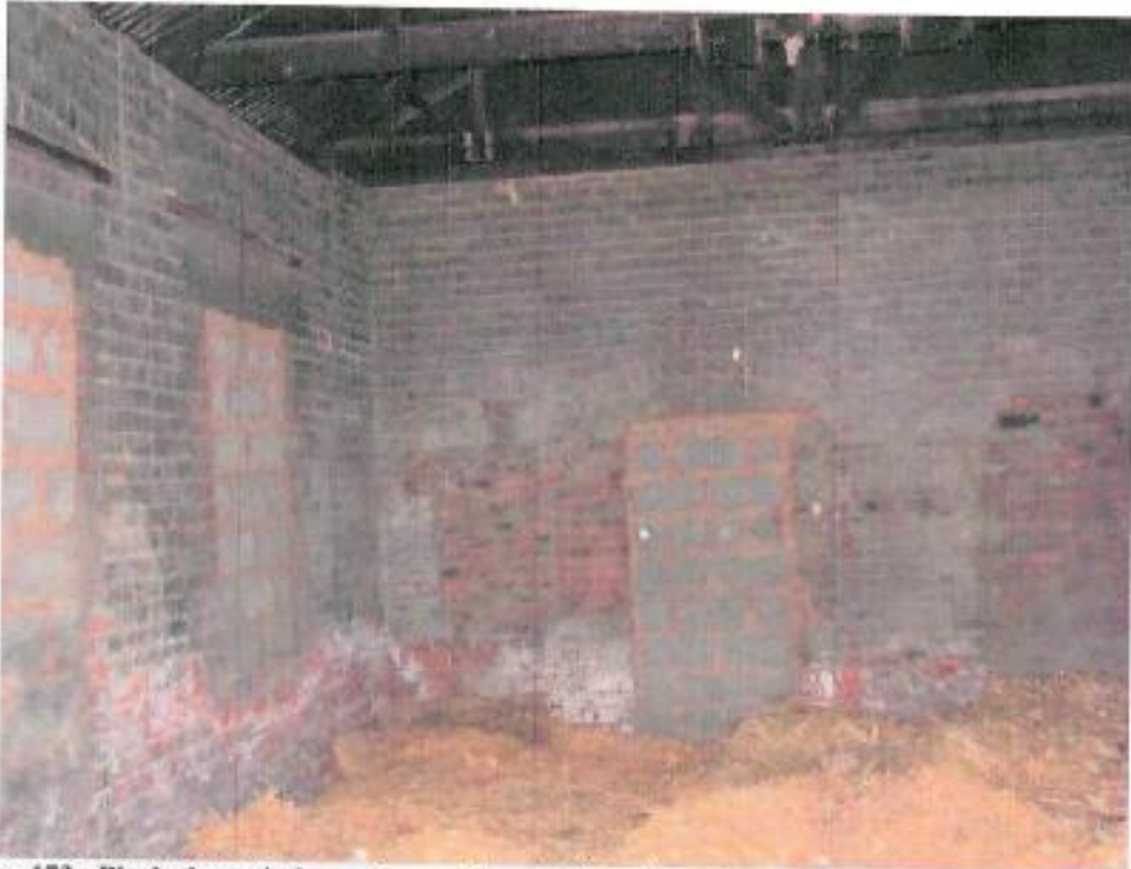
Figure 173: Blocked up windows – hay on floor indicate it could have been used for animal shelter or storage for animal feed
