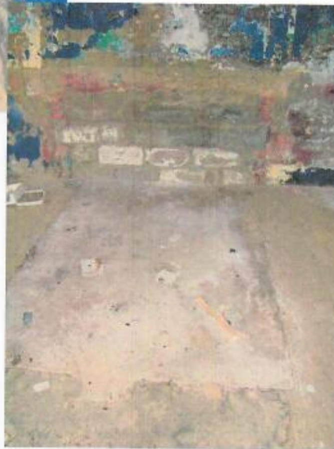
Figure 151: Blocked-up entrance of underground passage leading from Talley Room to the Change Room in the Treatment Plant area
