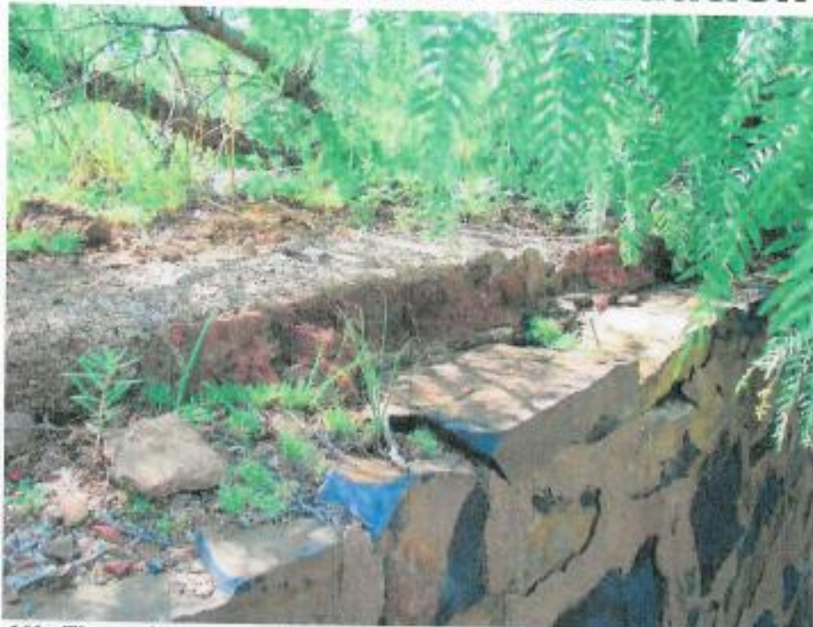
Figure 161: The north eastern section of this building has a stone foundation with a cement and brick layer on top
