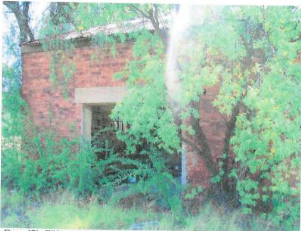
Figure 171: Wide entrance – appears to have been reinforced with cement at a later stage
