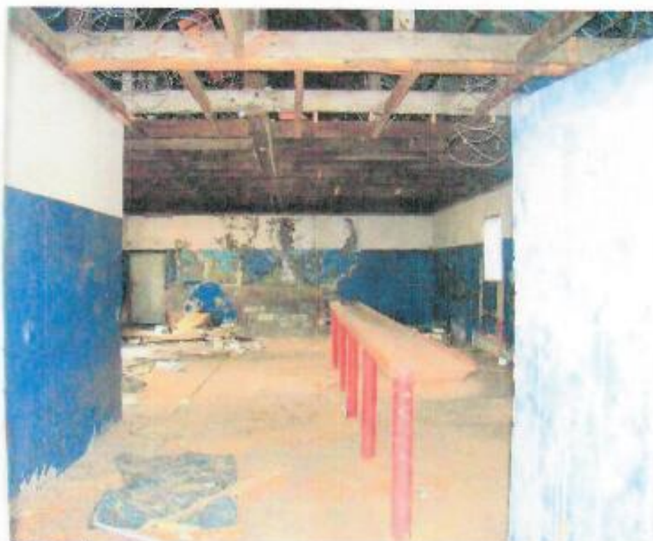
Figure 149: Interior of Talley Room (Door to the left leads to a passage that ends outside the hostel). Area in the middle of the back wall immediately to the left of the counter is the blocked up entrance to the underground passage)
