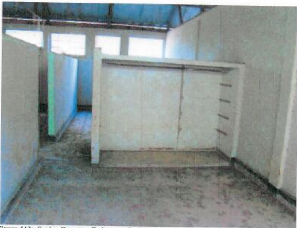
Figure 113: Senior Quarters Bedroom – built-in closet space divides this space into two rooms
