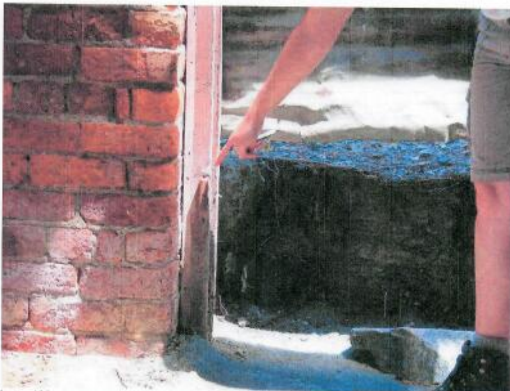
Figure 133: Photograph taken from inside Isolation Ward – note build-up of soil on the outside (southern side)
