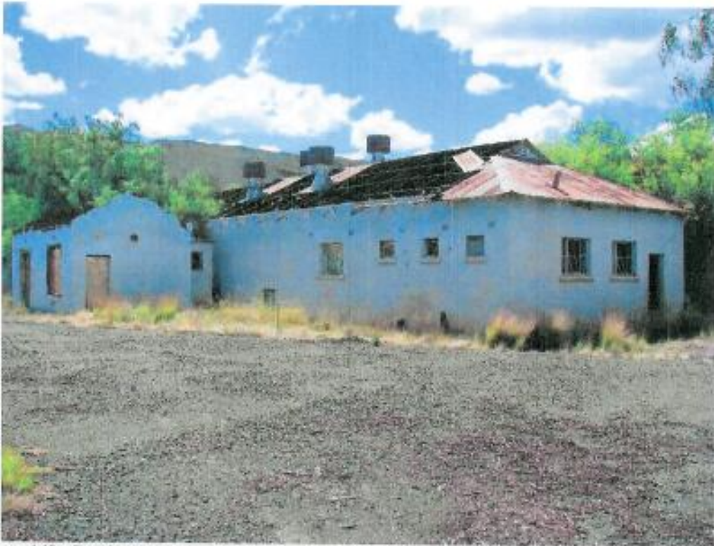
Figure 140: Southern exterior view of the hospital buildings (attached to main hostel) – orientation north-west
