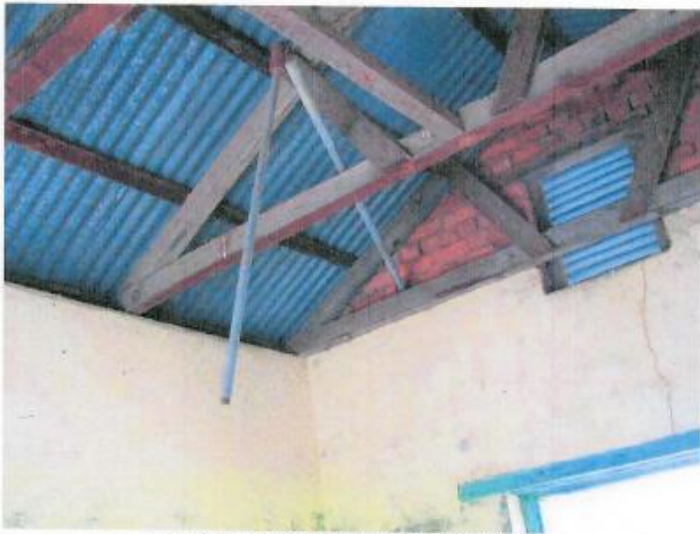
Figure 137: Water pipes suspended from ceiling
