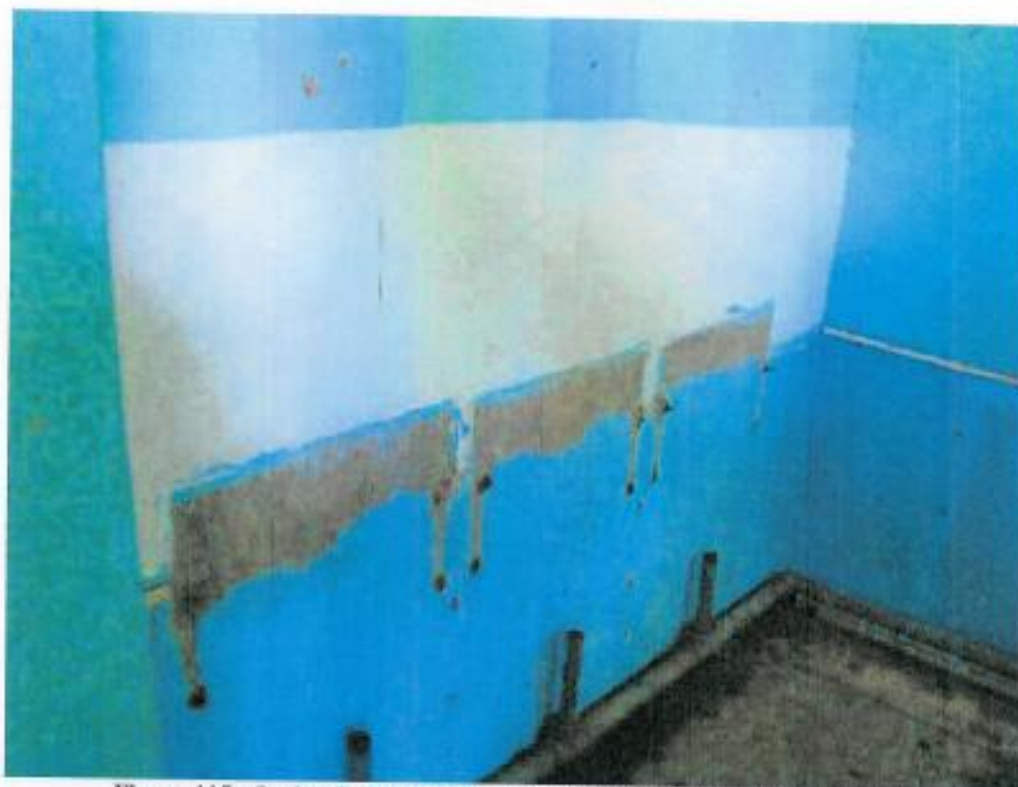
Figure 115: Senior Quarters bathroom (area where basins were affixed)
