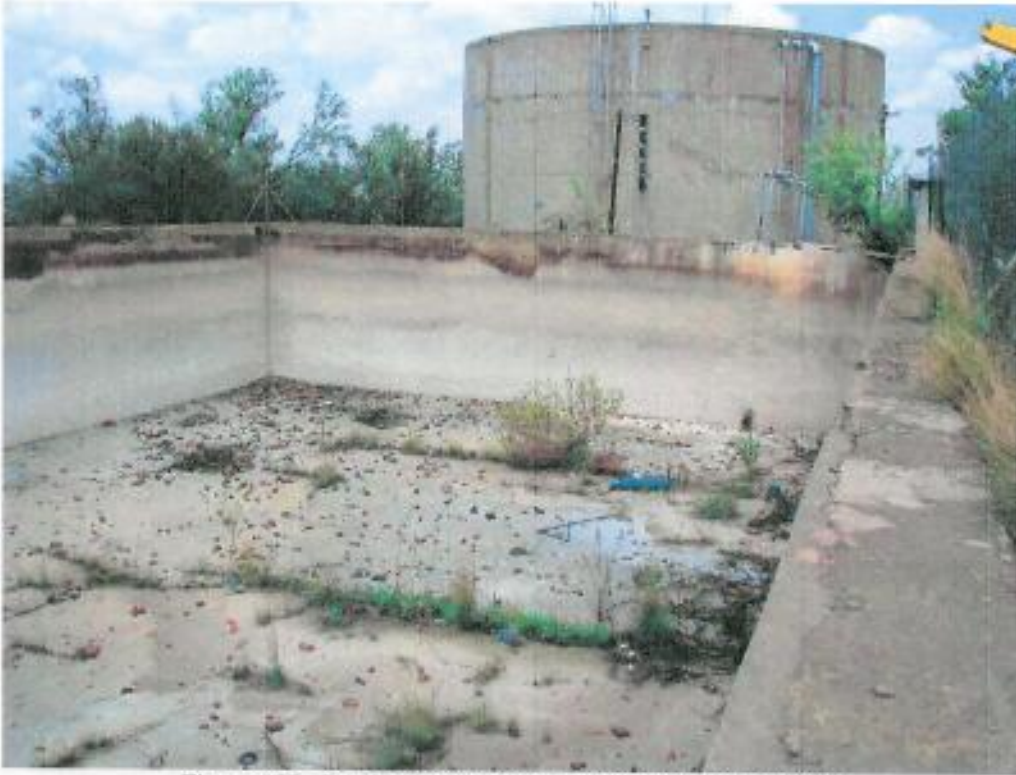
Figure 155: Potable storage tank in back, reservoir in front
