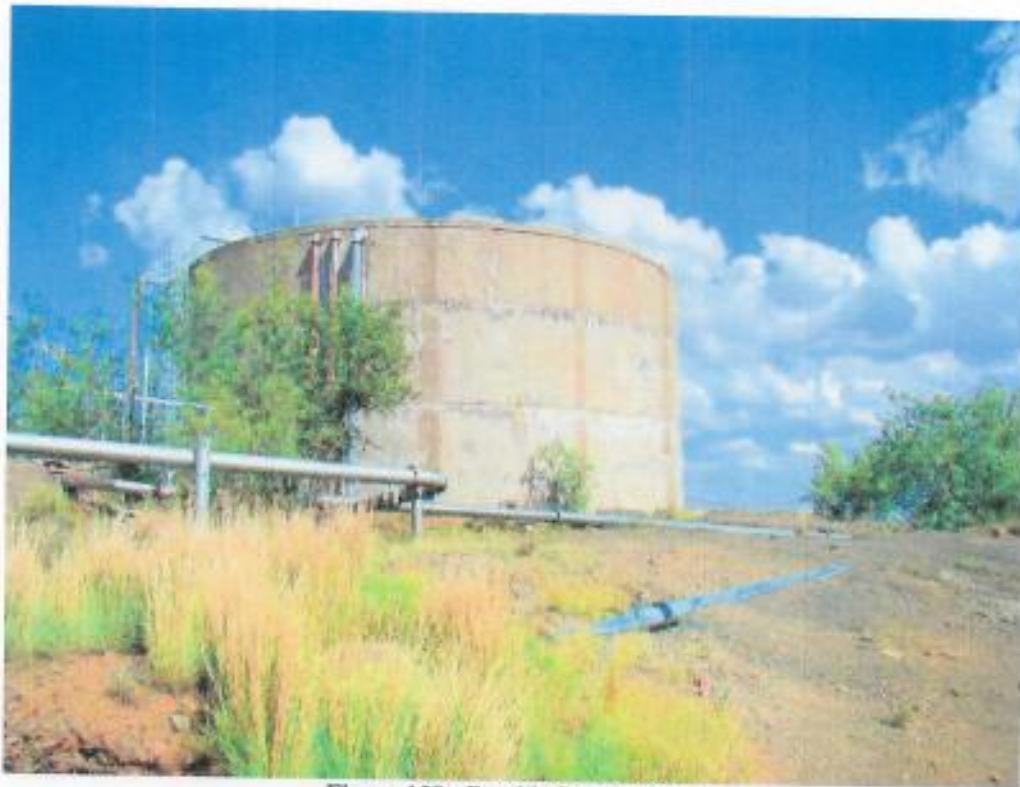
Figure 158: Potable Storage tank
