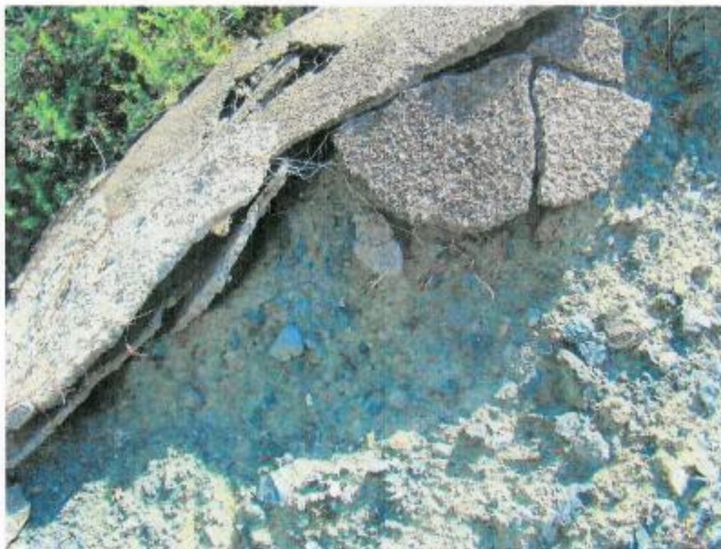
Figure 226: Close-up view shows the mesh with thin layer of cement on top
