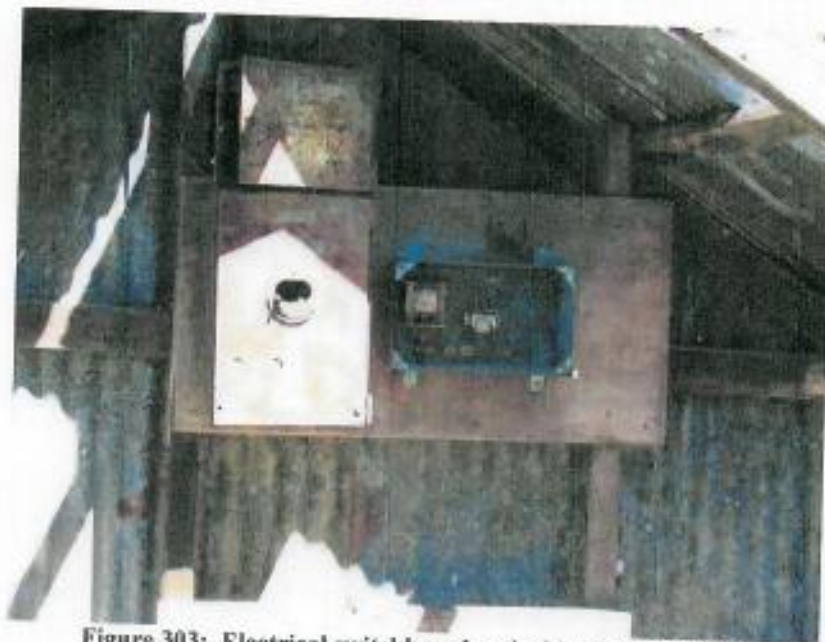
Figure 303: Electrical switchboard on inside of pump house
