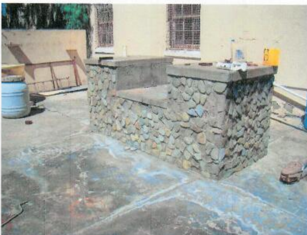
Figure 346: The barbeque facilities were added during the time the hall was used as "Moth Hall"
