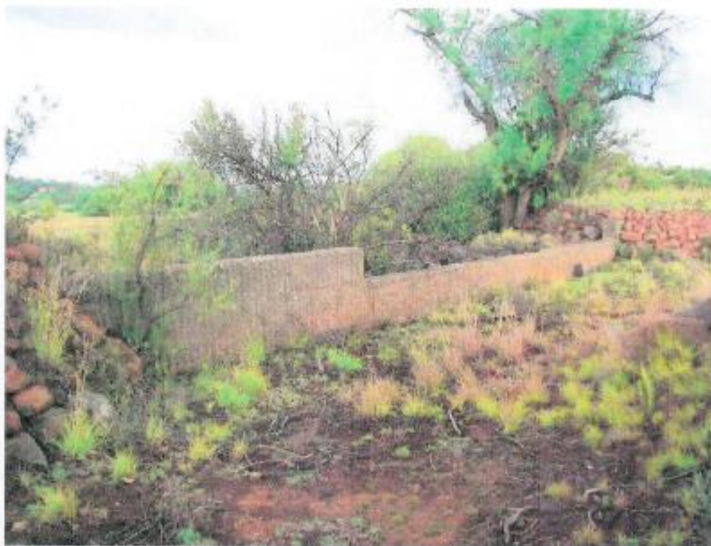
Figure 371: A cement retainer wall in a ditch (sides of ditch packed with stone) – orientation north-west
