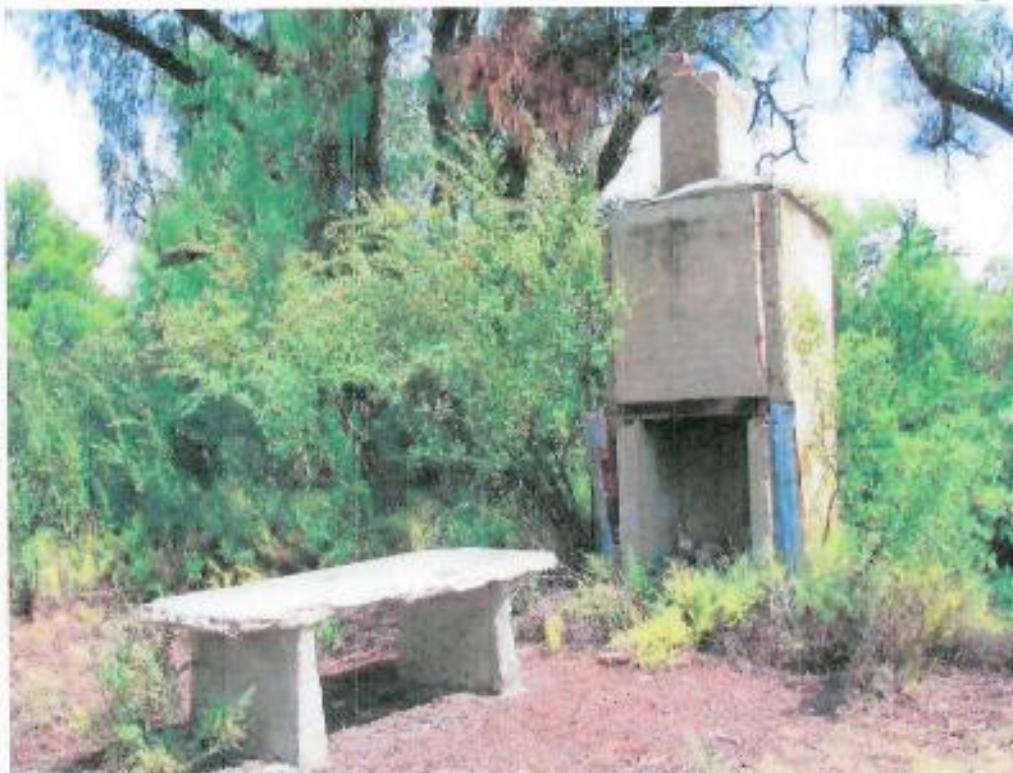
Figure 334: Chimney and table remains
