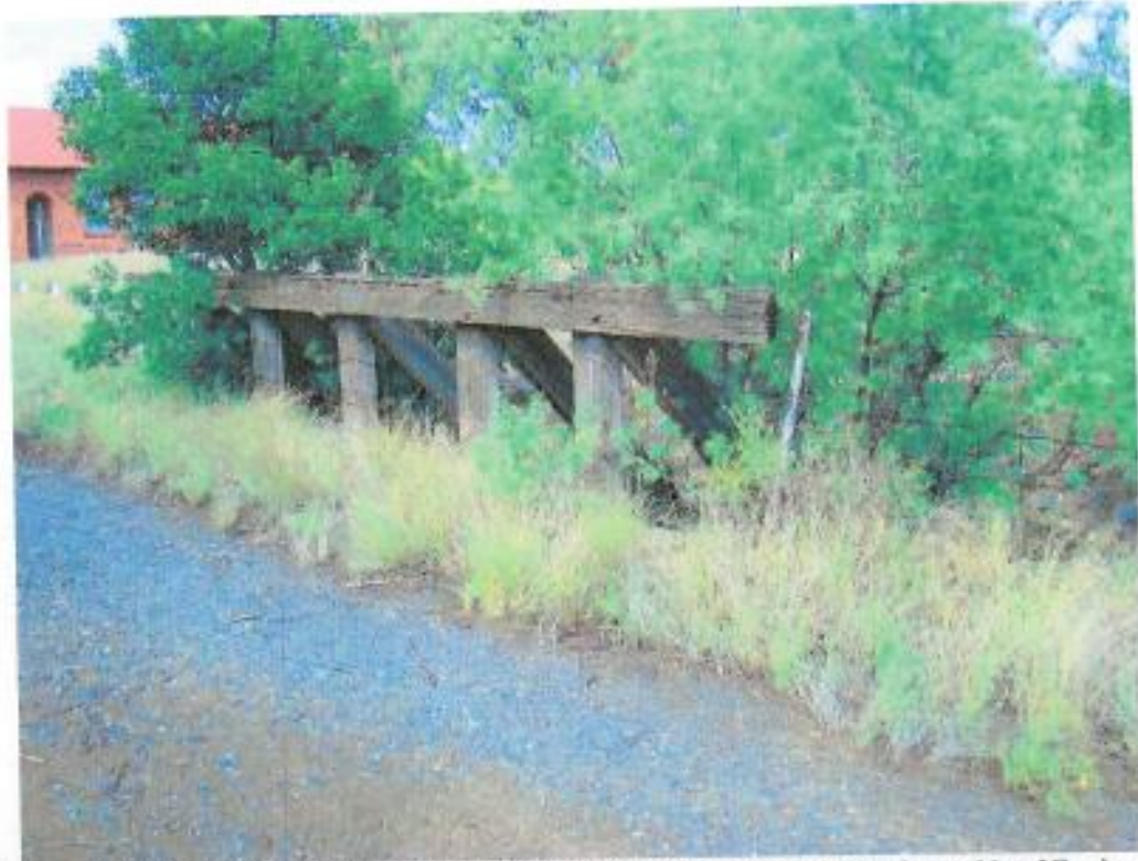
Figure 448: Bridge leading to unidentified structure no 25 on map on southern side of Engineers Office
