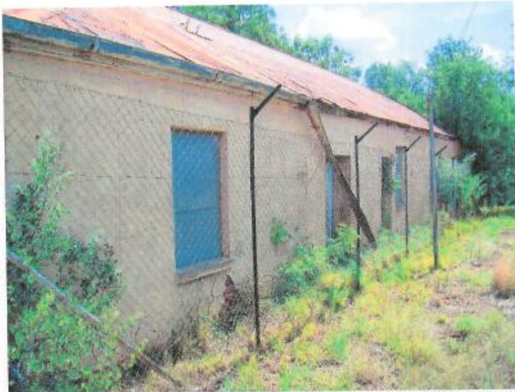
Figure 458: Unidentified structure indicated as mine building on earlier maps (see position 1 on map)
