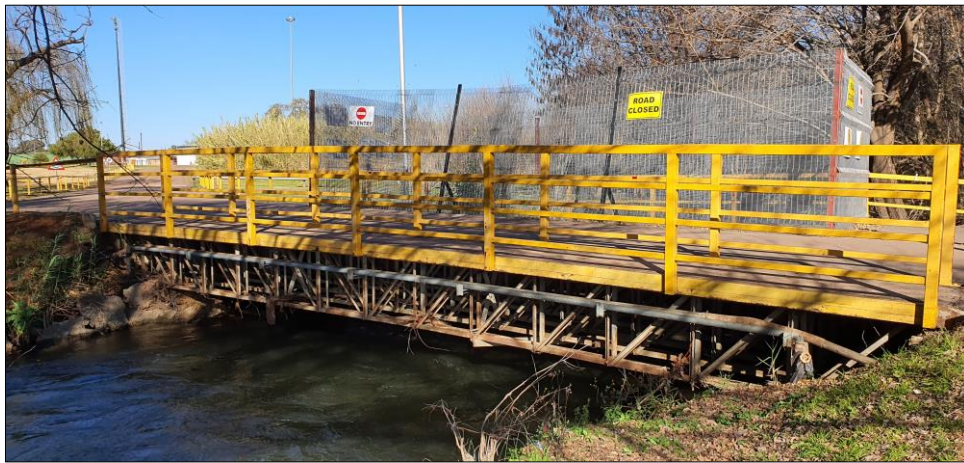
Figure 13: General view of the unstable bridge
