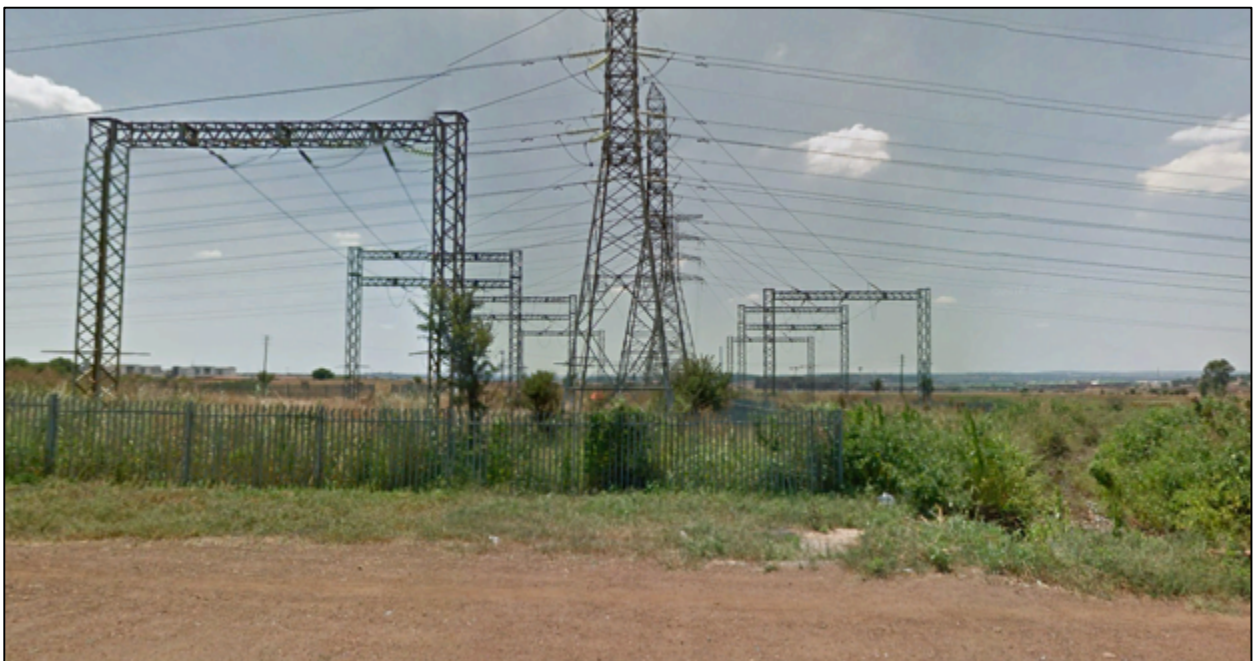
Figure 22. Power Station adjacent to Nelmapius Drive
