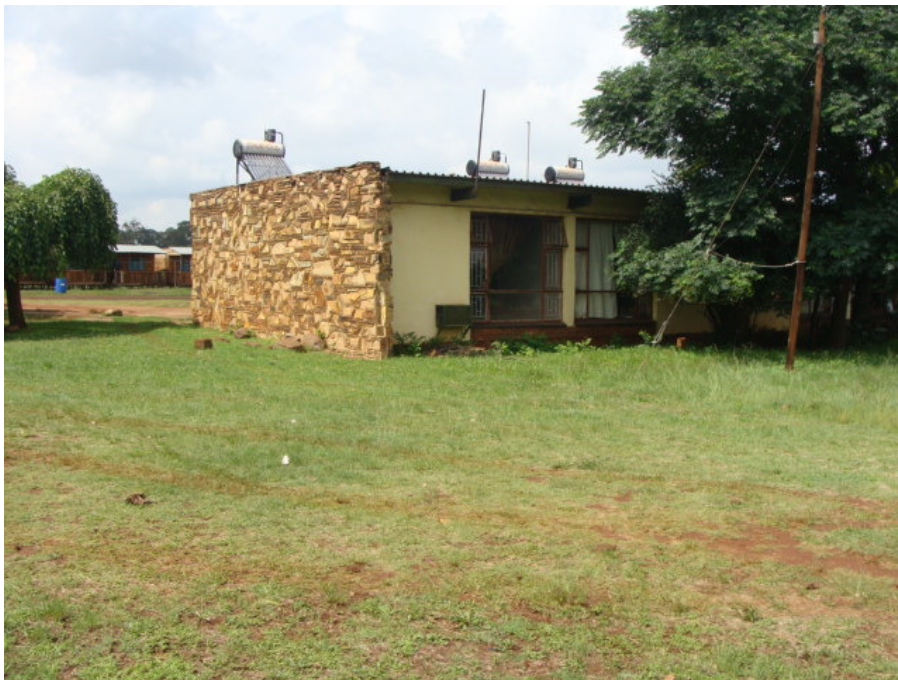
Figure 15 Another section of rooms of the hotel dating to ca. 1960, but showing later changes.
